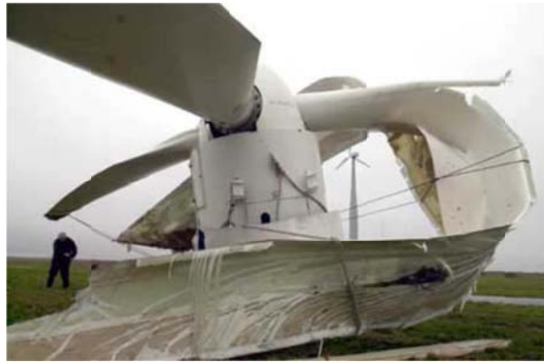
Figure 15: Catastrophic wind turbine failure (12).
