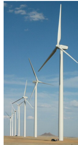
Figure 1. GE 1.5 MW Wind Turbines in the Colorado Green wind farm near Lamar, Colorado. The item at the base of the closest turbine is a minivan.
