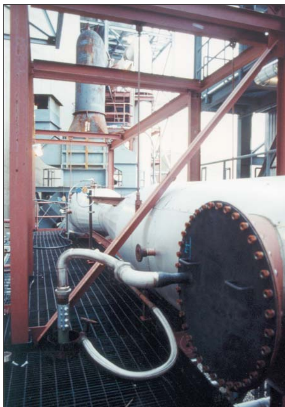
The sorbent injection into the duct upstream of SO x -NO x -Rox Bag TM system.
