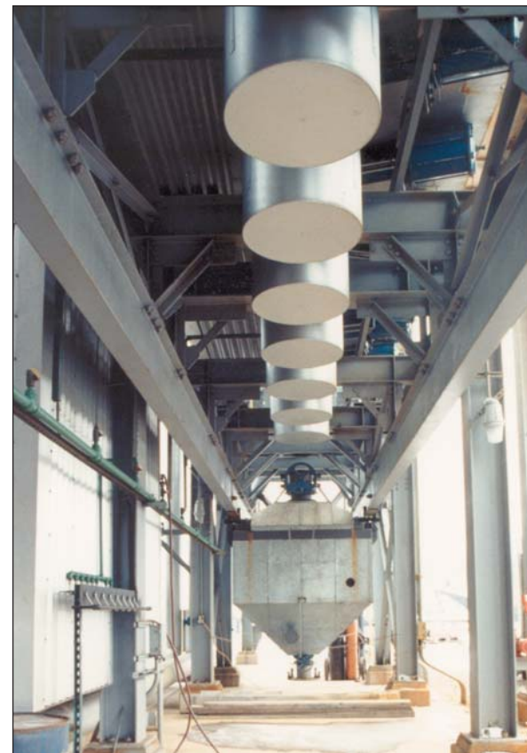
The bottom portion of the SO 2 converter reactor, with the catalyst dust collector hopper mounted on steel rails (center).
