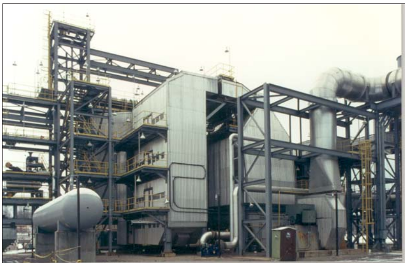
The SNOX™ demonstration at Ohio Edison's Niles Station Unit No. 2 achieved SO 2 removal efficiencies exceeding 95% and NO x reduction effectiveness averaging 94%. Ohio Edison is retaining the SNOX™ technology as part of its environmental control system.
