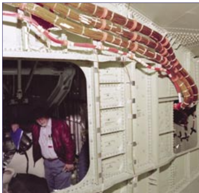
Figure 4.2-3. Typical wiring bundle inside Orbiter wing.
