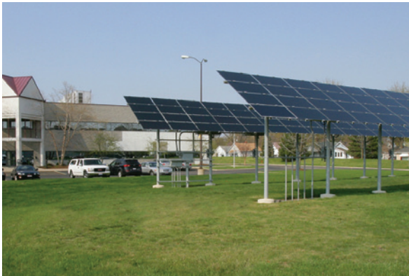
A visit to the University of Toledo's Clean and Alternative Energy Incubator was part of the recent Forum on Energy Efficiency in Manufacturing, a one-day event organized by the Department of Commerce. The event was part of the department's effort to promote the competitiveness of U.S. manufacturers. (photo courtesy University of Toledo)
