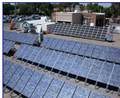
Figure 1 A portion of the PV arrays at DETL.
