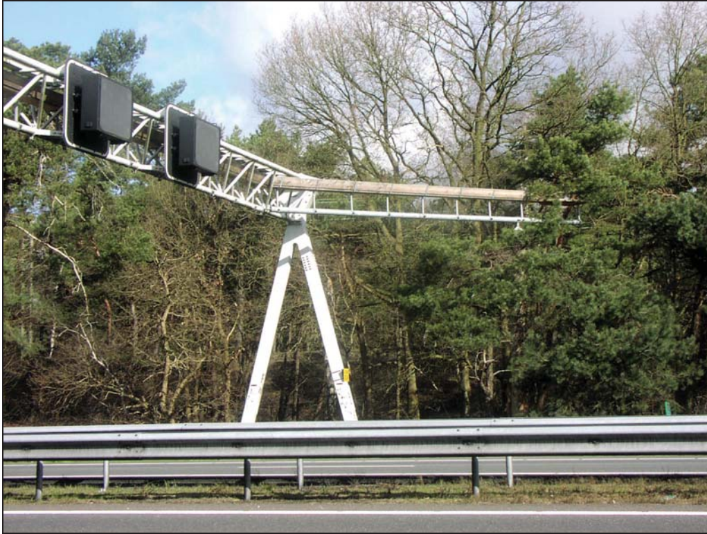
Figure 37. Photo. Canopy crossing installed in permanent signage fixture (Credit: Tony Clevenger).
