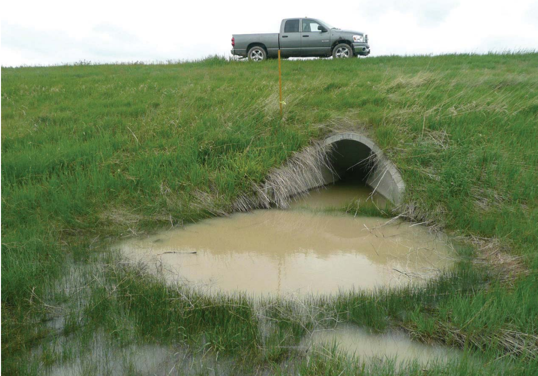
Figure 58. Photo. Flooding in front of tunnel due to improper drainage design (Credit: Tony Clevenger).
