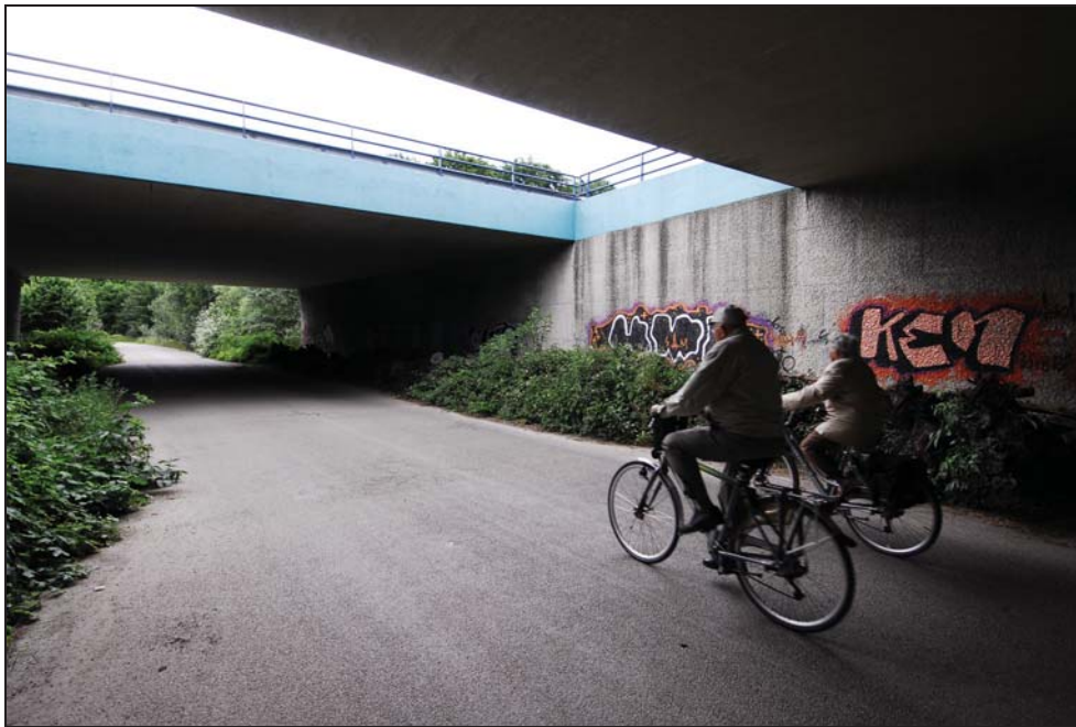
Figure 45. Photo. Multi-use underpass in The Netherlands retrofitted for human use and wildlife passage (Credit: Marcel Huijser).
