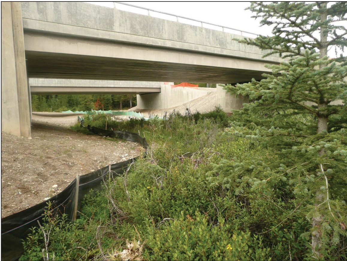
Figure 46. Photo. Wildlife underpass designed to accommodate waterflow (Credit: Tony Clevenger).
