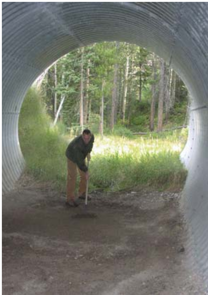
Figure 76. Photo. Raking of track bed in culvert Banff National Park, Alberta (Credit: Tony Clevenger/WTI).
