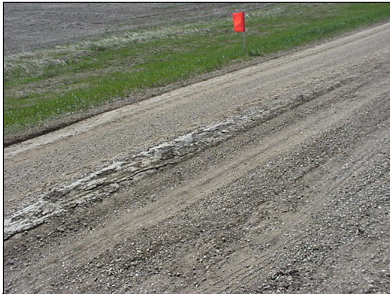
Rutting of gravel road.
