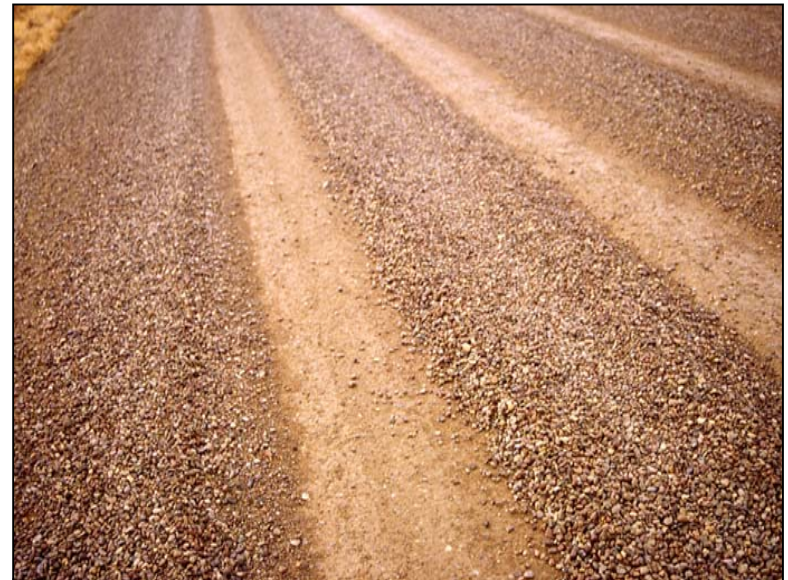
Gravel loss in wheel paths.
