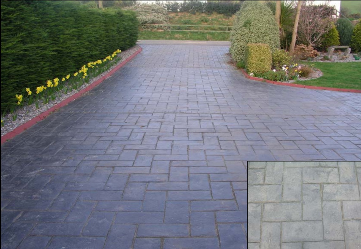
Stamped PCCP entranceway.
