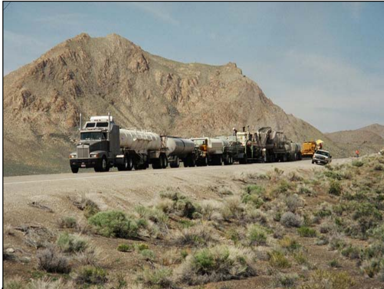
CIR equipment train.
