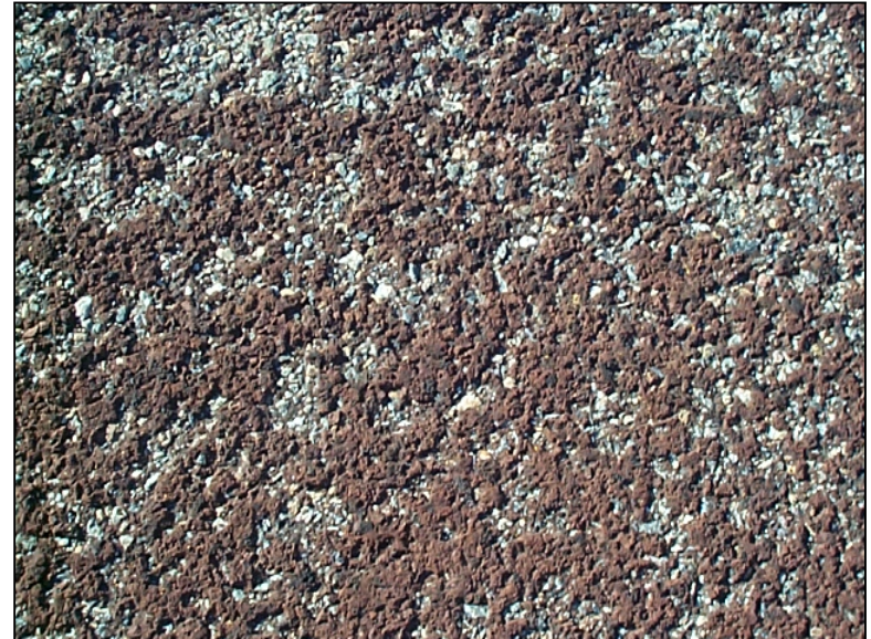
Worn chip seal surfacing with colored chips.
