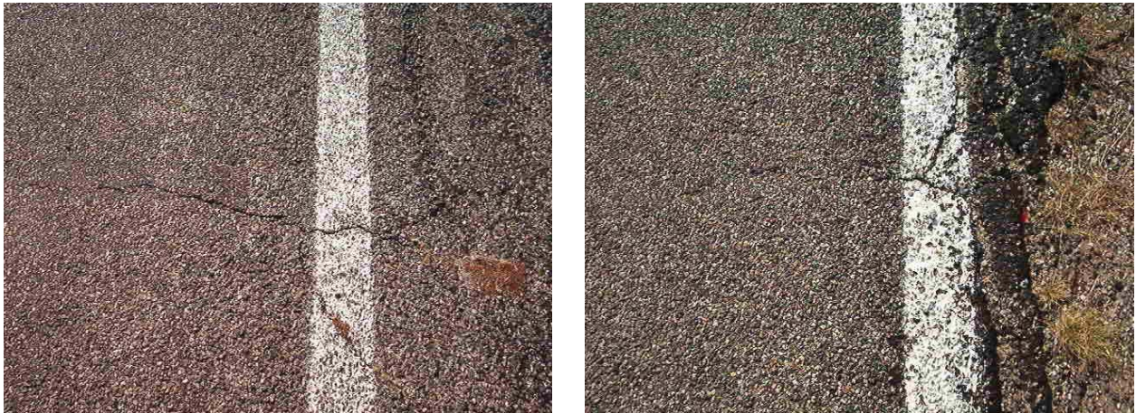
Figure 37. Photo. Examples of Cracks at Site 2.
