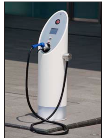
Electric vehicle charging station
