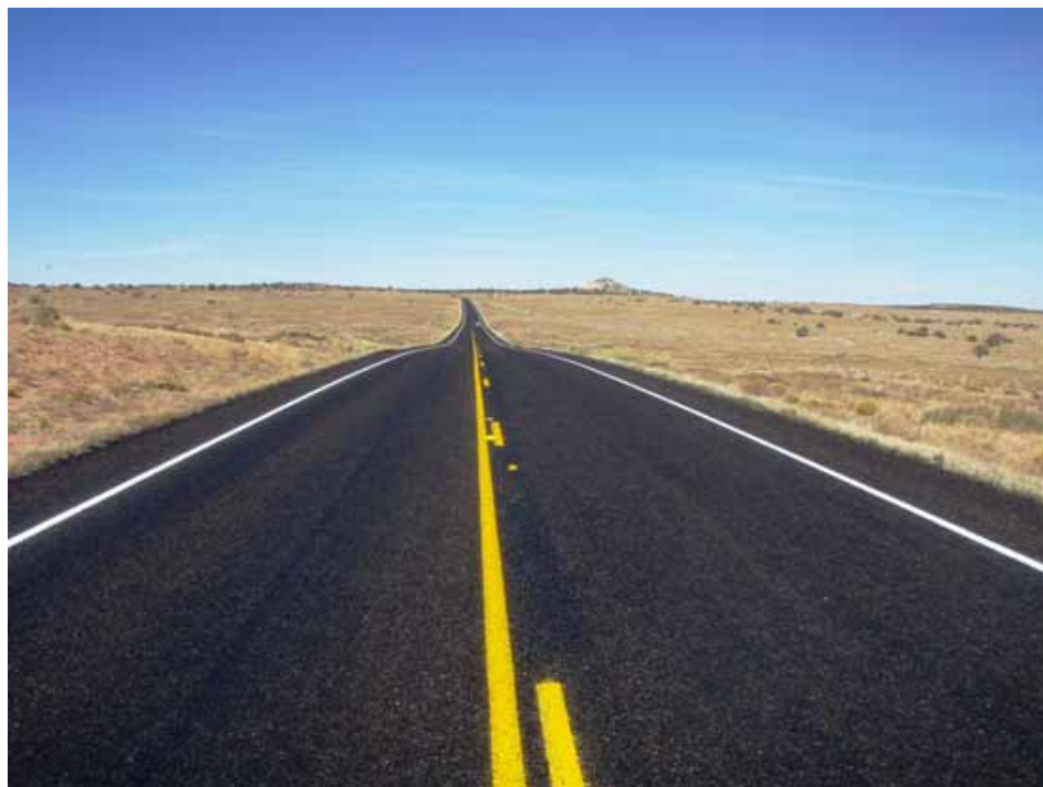
Figure 39. Photo. Utah Parks Project—Canyonlands NP Finished Chip Seal after Fog and Striping.
