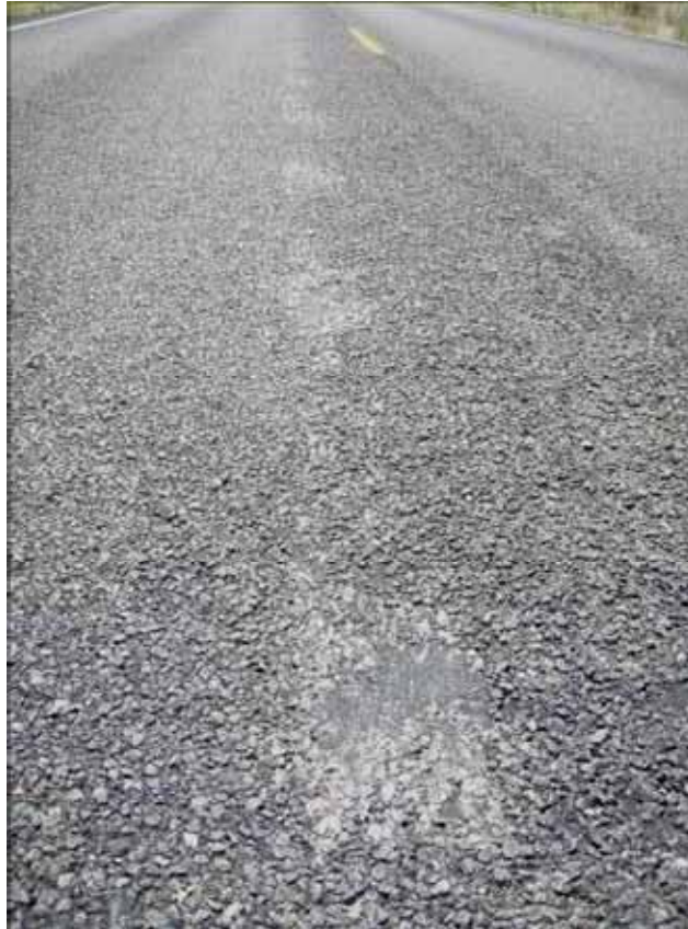
Figure 84. Photo. Utah Parks Snow Plow Damage in July 2009.
