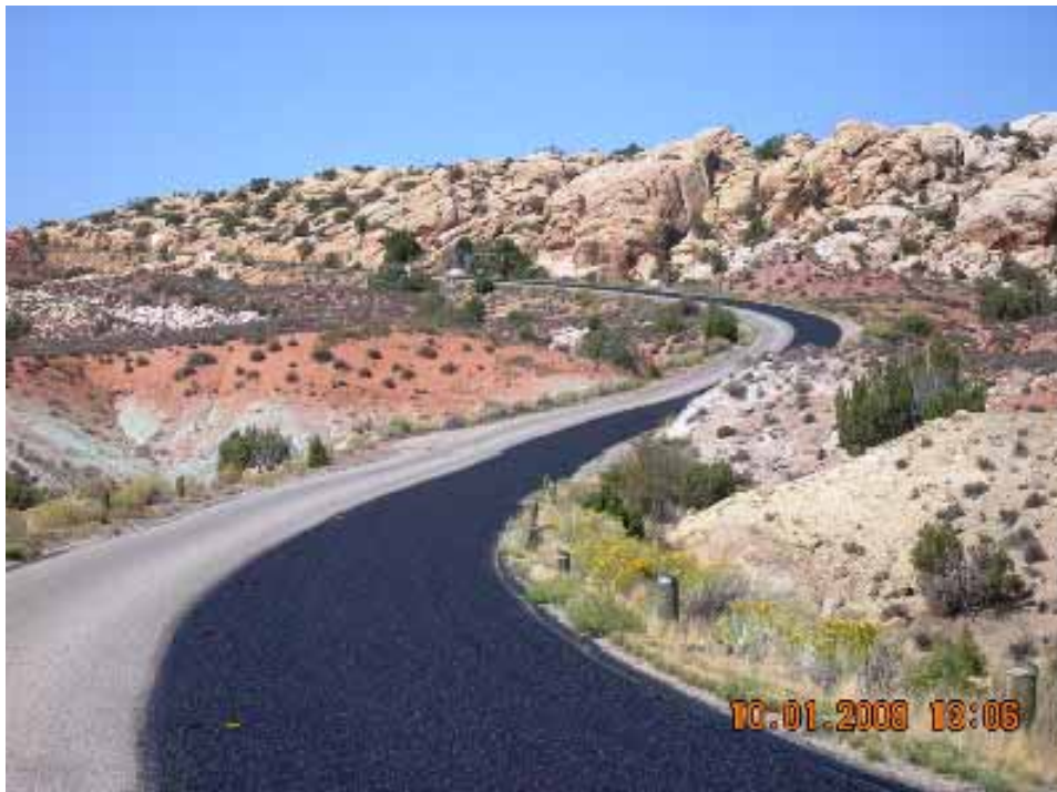
Figure 35. Photo. Utah Parks Project—Arches NP Partially Fogged.
