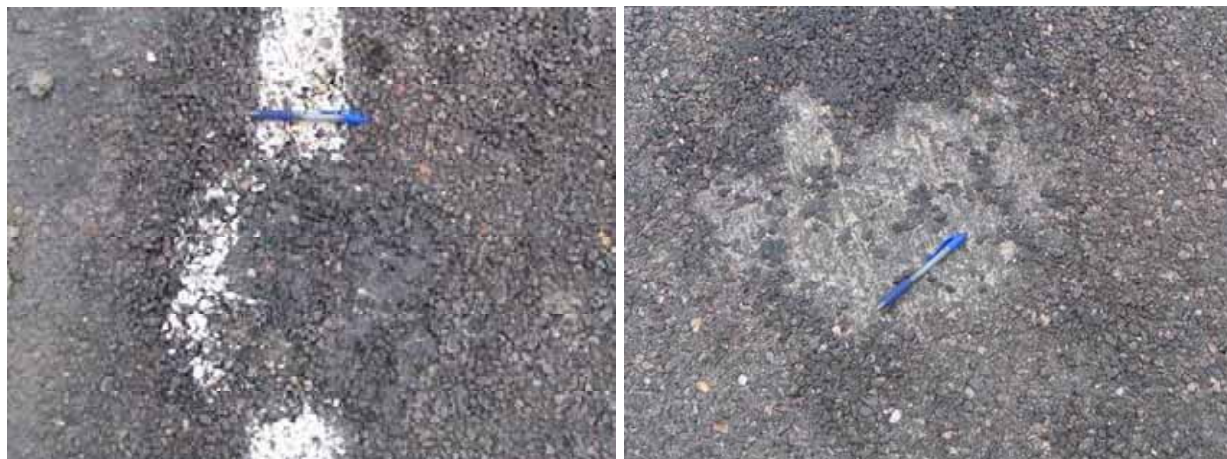
Figure 86. Photo. Wearing and Chip Loss on Dinosaur Project in July 2009.
