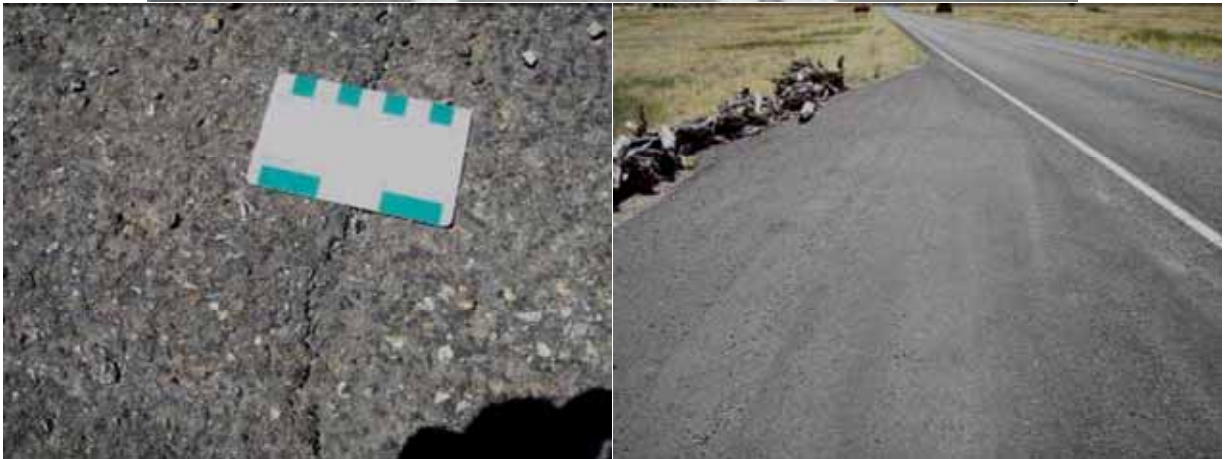
Figure 83. Photo. Utah Parks Micro Surfacing in July 2009.
