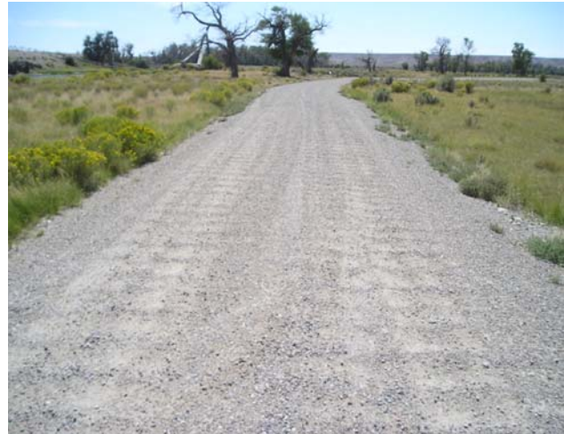
Figure 12. Photo. Section IV Washboarding.
