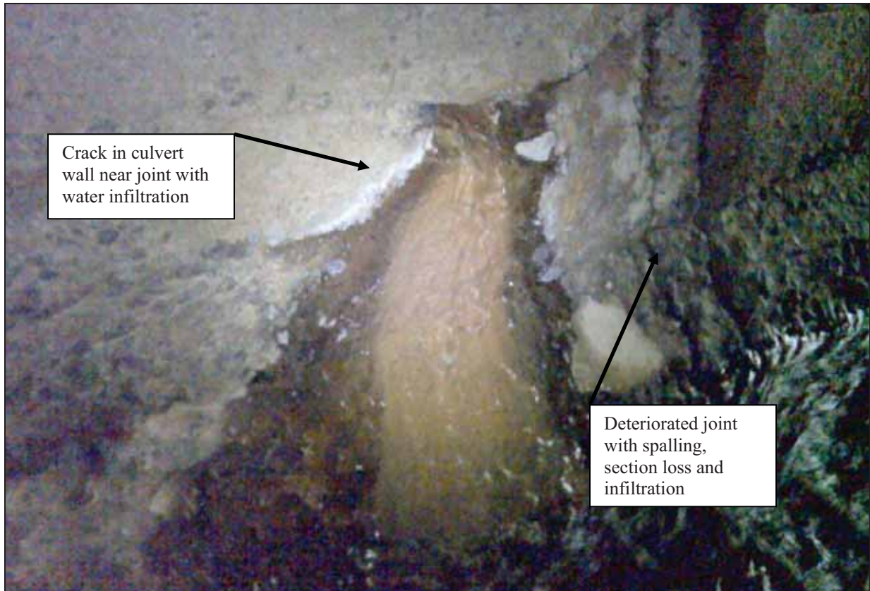
Figure 39. Photo. Diagonal crack near joint and invert with water infiltration .
