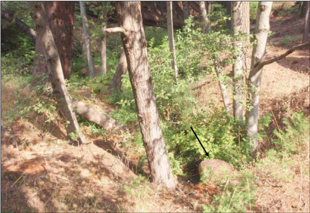
Figure 47. Photo. Stable downstream channel conditions at the outlet of CMP example in Yosemite National Park.
