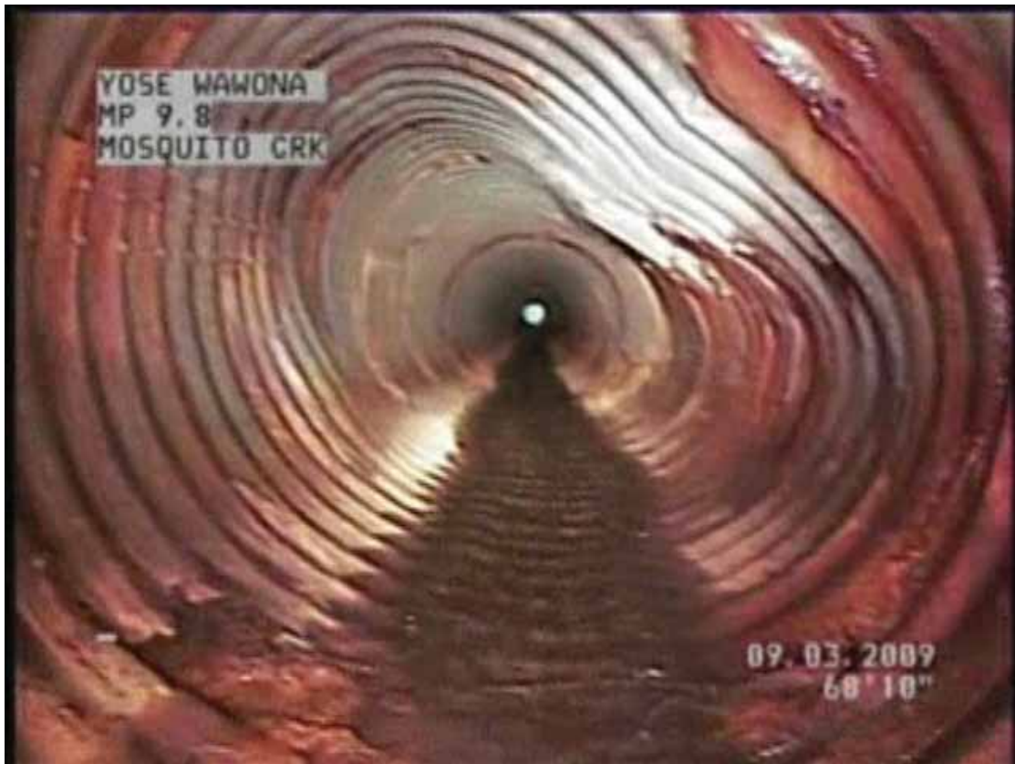
Figure 51. Photo. ROV video of CMP example showing deformation and invert section loss.
