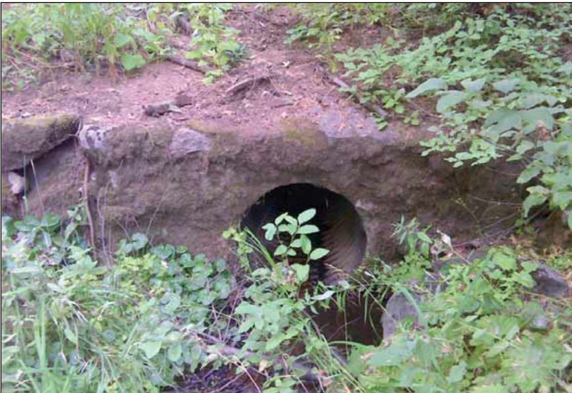
Figure 46. Photo. Light invert deterioration at inlet of CMP example on Mosquito Creek in Yosemite National Park.
