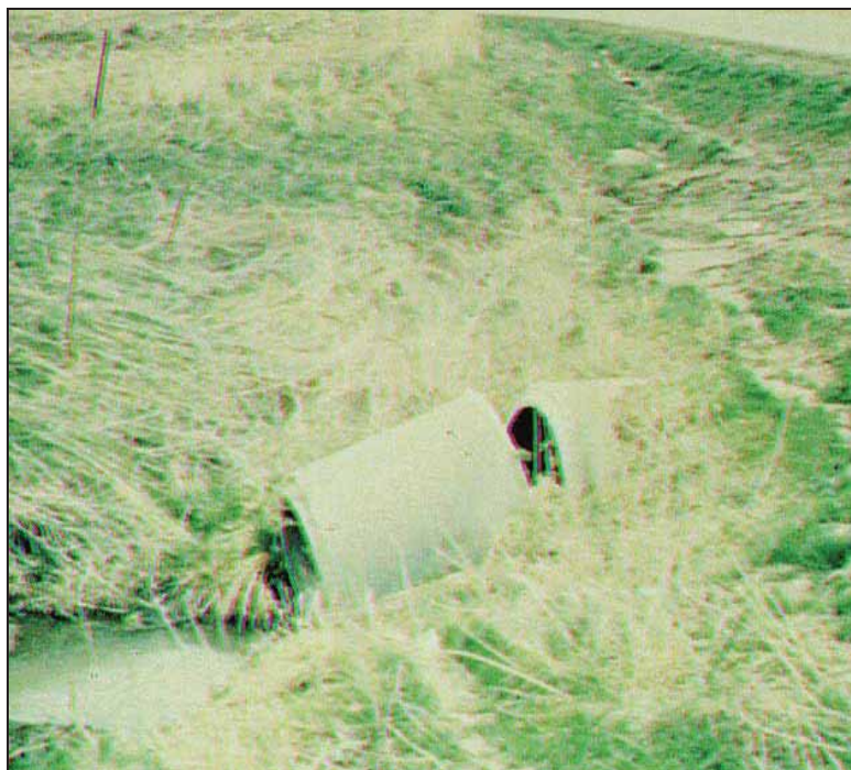
Figure 8. Photo. RCP culvert damaged by scour. (2)
