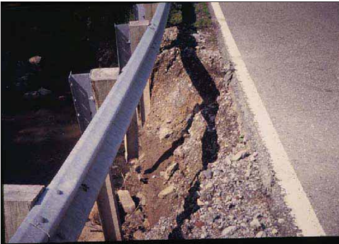
Figure 6. Photo. Erosion damage to downstream embankment slope and shoulder from previous overtopping. (3)
