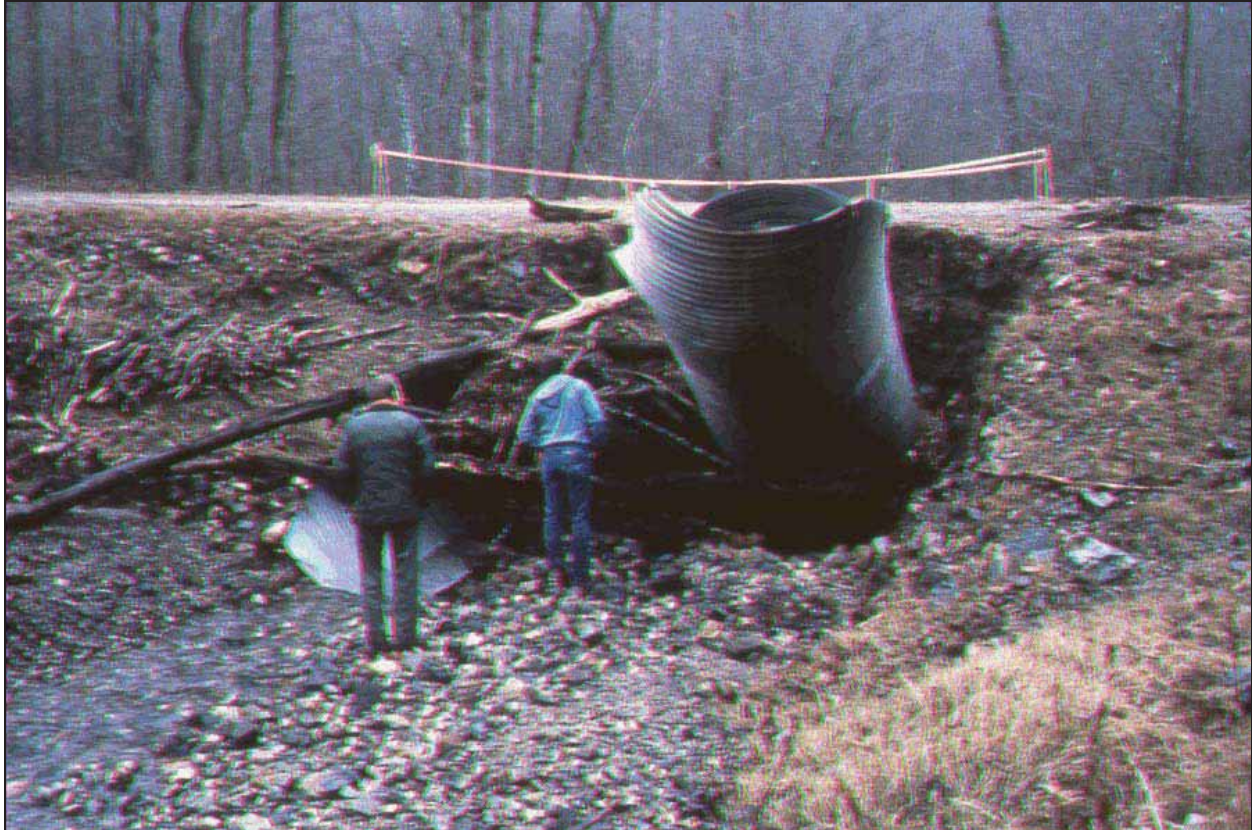
Figure 4. Photo. Example of severe buoyancy uplift (FHWA/NHI training materials). (2)
