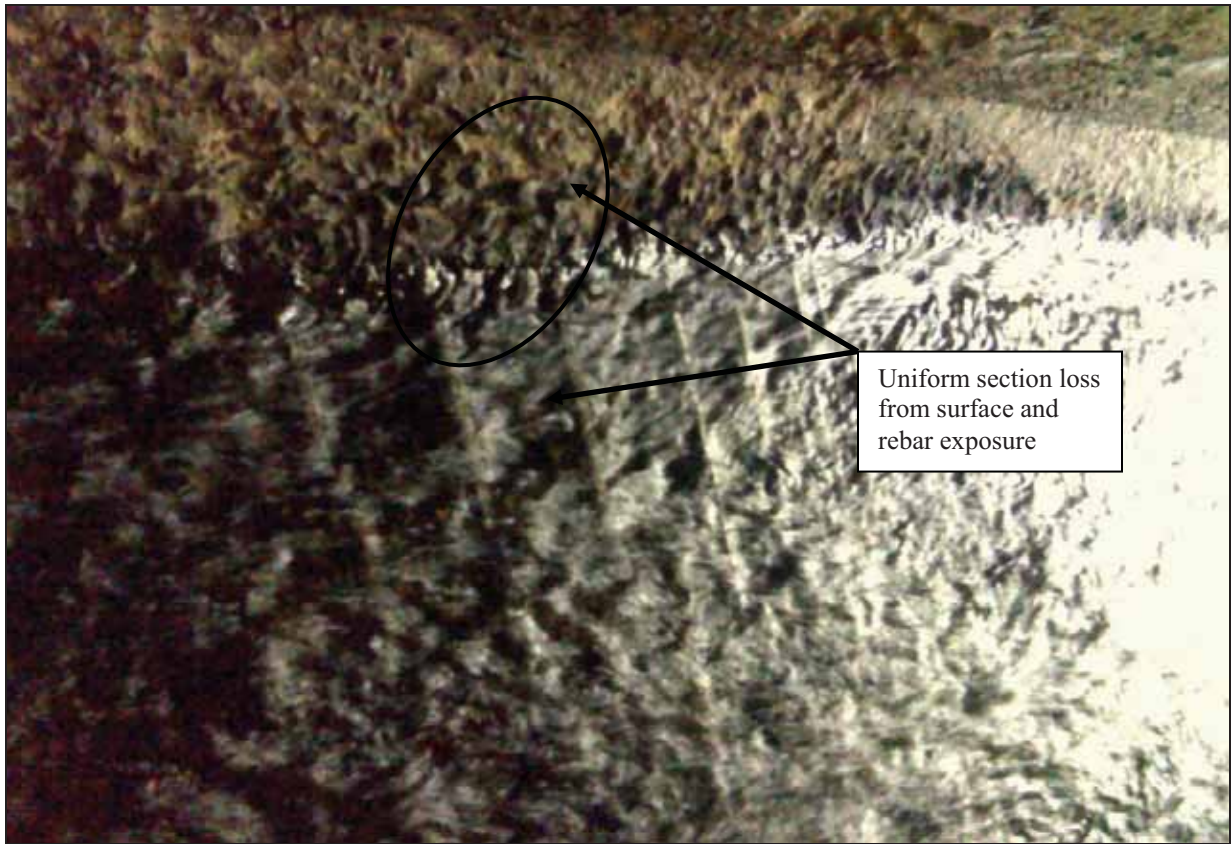
Figure 37. Photo. Invert abrasion damage with concrete section loss and exposed/corroding rebar.
