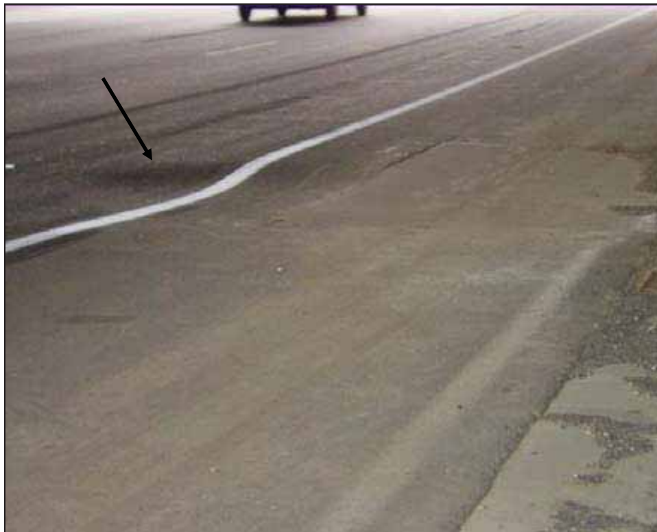
Figure 11. Photo. Example of roadway settlement caused by voids around a culvert. (3)
