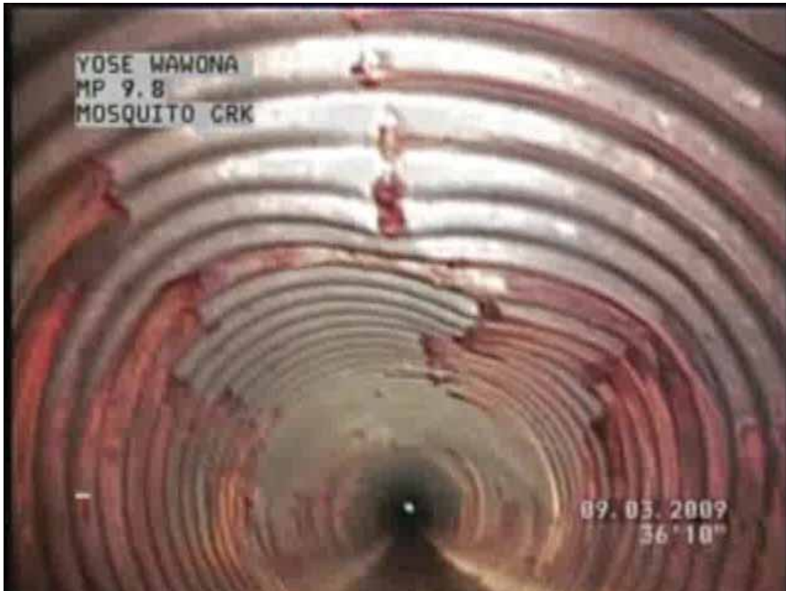
Figure 50. Photo. ROV video of CMP example showing crown deformation and cracking.
