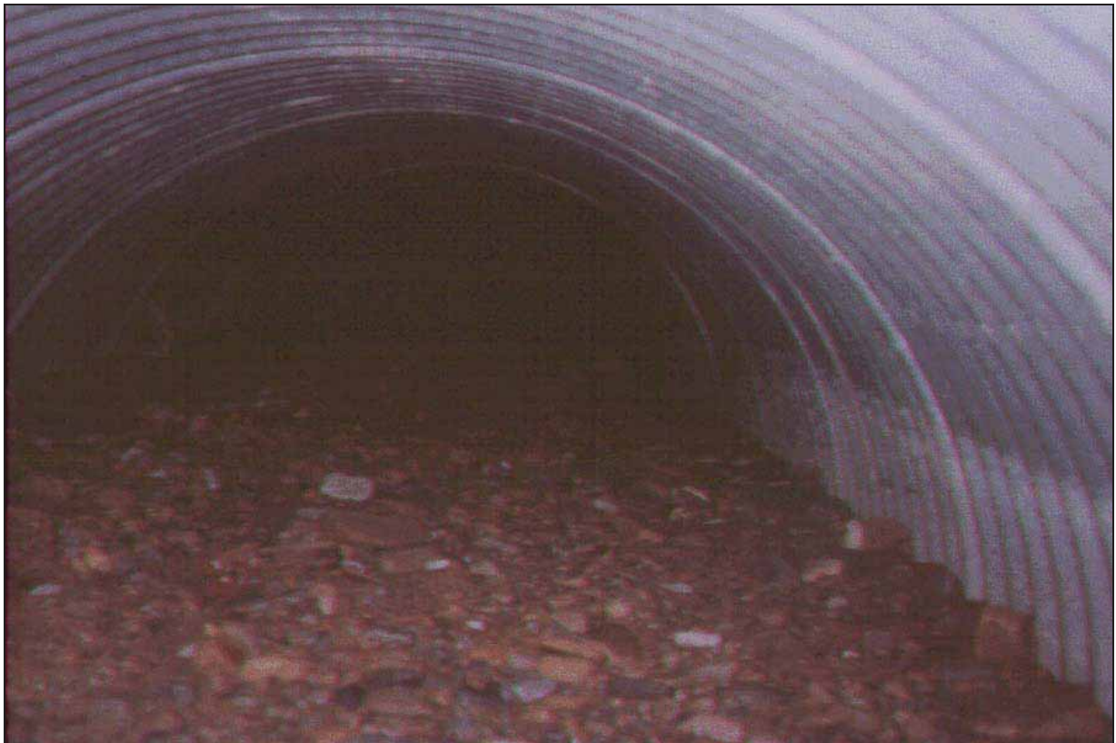
Figure 14. Photo. Culvert barrel filled with sediment up to half its rise, possibly due channel aggradation. (2)
