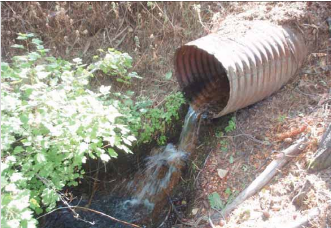
Figure 45. Photo. Light invert deterioration and minor local scour erosion at outlet of CMP example.
