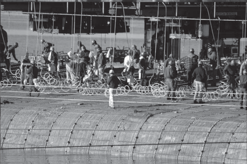
Mats are tied together using pneumatic tying tools and launched in front of the New Orleans District.
