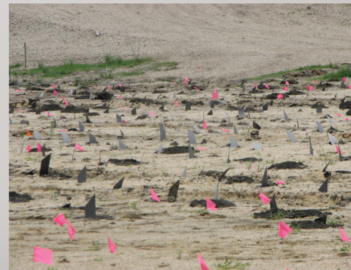
Wick drains help increase the strength of the underlying soil by removing excess sub-surface water. USACE Photo by Nick Silbert
