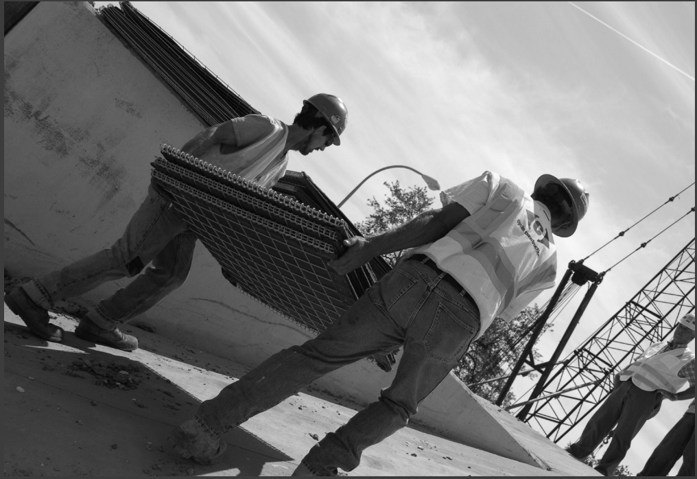
Above: Prior to Hurricane Isaac's landfall, crew members place HESCO baskets at the Leroy Johnson floodgate to close construction gaps. (Photograph by Paul Floro)
