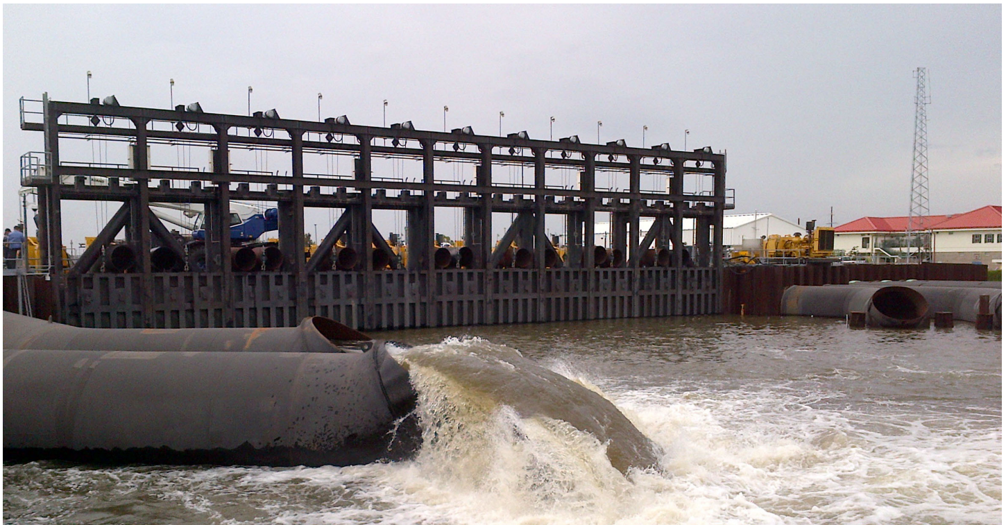
Below: The gates at the 17th Street Outfall Canal Interim Closure Structure were closed against rising water levels in Lake Pontchartrain and pumps were used to evacuate interior drainage water from behind the gates. (Photo by Paul Floro)
