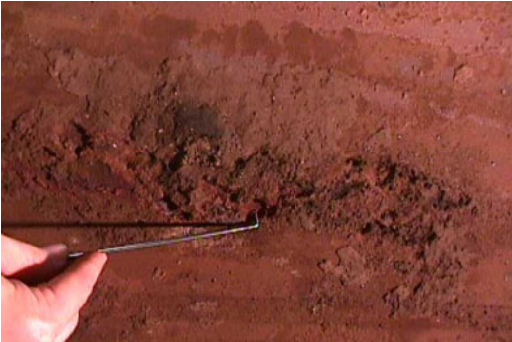
Figure 8. Corrosion pitting on inside of pipe near rupture site.
