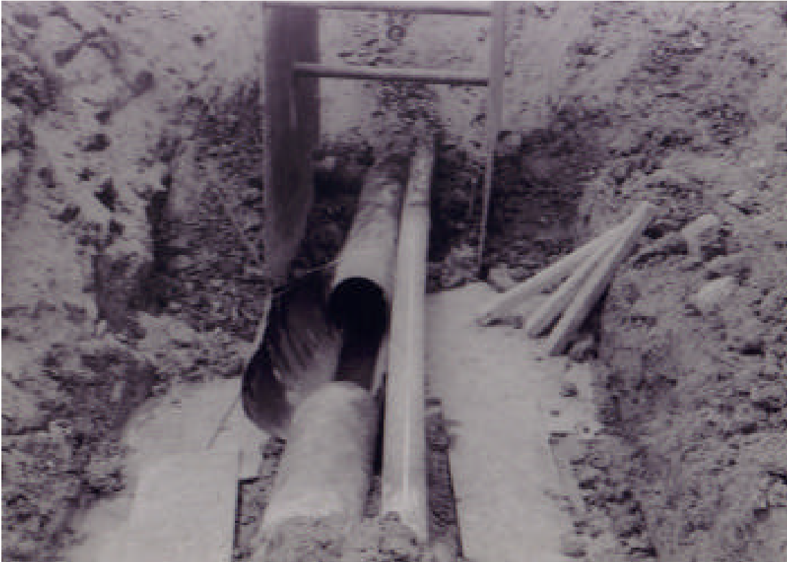
Figure 1. Postaccident excavation revealing relative positions of 8-inch distribution main and 20-inch transmission pipeline at site of rupture
