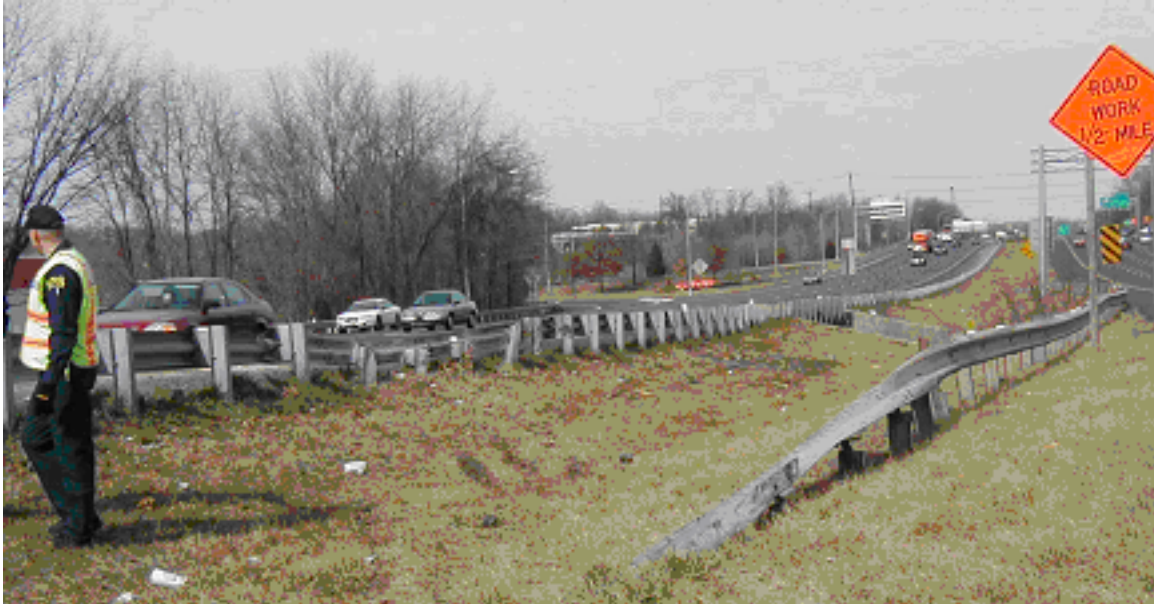
Figure 11. Explorer path down the northbound cross slope, over the turned-down guard-rail end treatment, through the depressed earthen median, and over the backside of the southbound guardrail.
