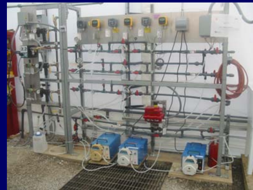
Skid with pumps and meters for wells inside Big Top
