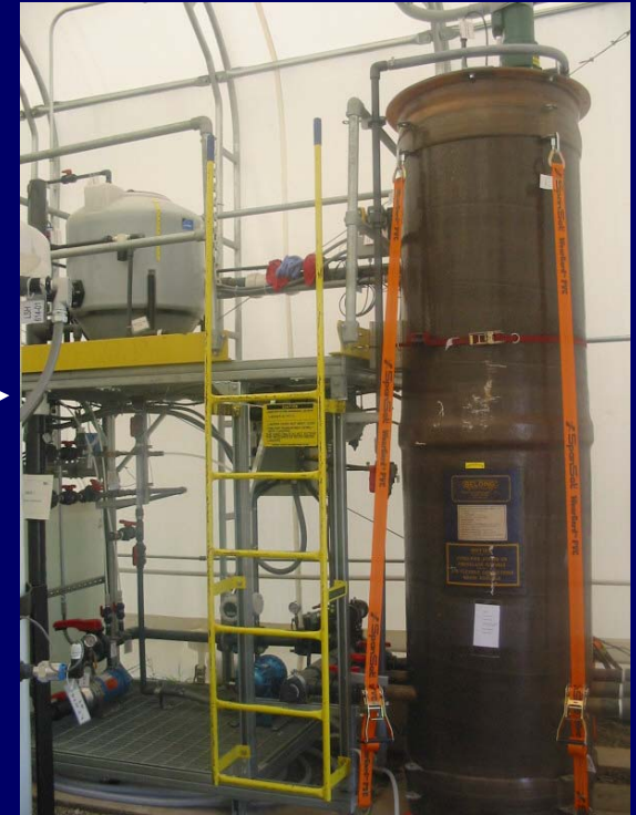
Fluidized bed reactor (FBR)
