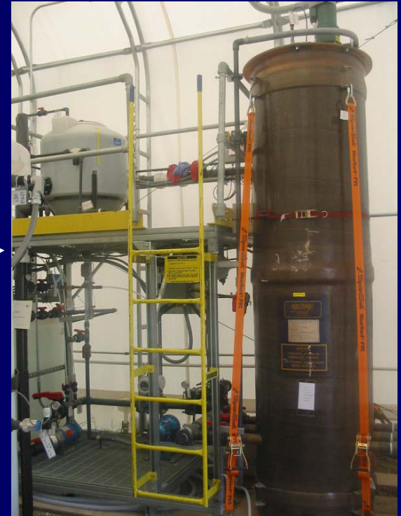
Fluidized bed reactor (FBR)
