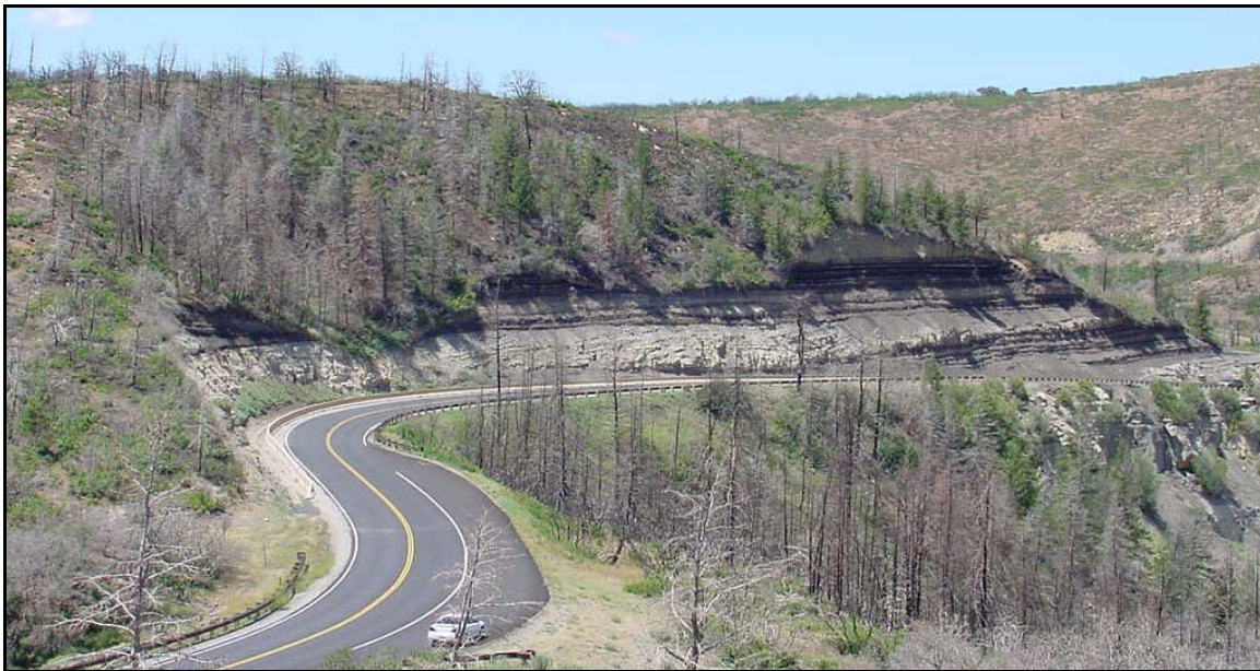
Figure 18. Photo. Unstable slope near Mile Post 9.3 in Mesa Verde National Park, CO.
