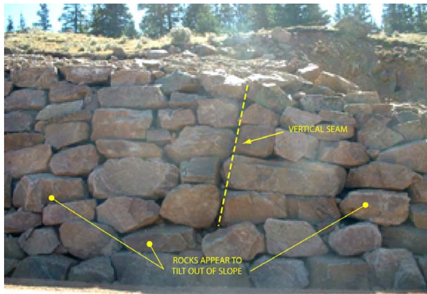
Figure 75. Photograph. Example of improper rockery layout evidences by vertical seams and rocks inclined out of face.
