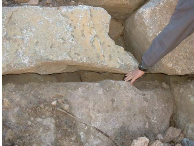
Figure 68. Photograph. Example of an unacceptable rock bearing.
