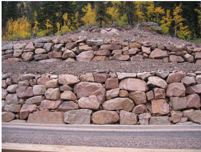
Figure 67. Photograph. Example of a relatively well constructed rockery.
