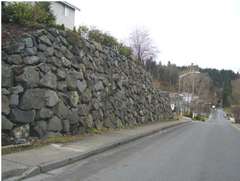
Figure 12. Photograph. Two-tier, 7.3-m (24-ft) rockery, 15th Avenue at 12th Street, Puyallup, Washington (Site 2), with guy wire anchored at base of rockery.
