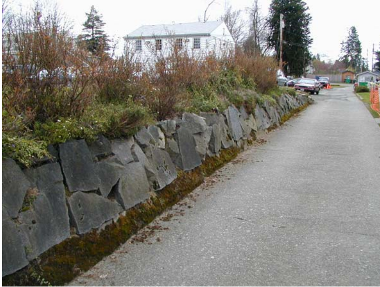
Figure 13. Photograph. Single-tier, 1.2-m (4-ft) rockery near state capital building, Olympia, Washington (Site 3).
