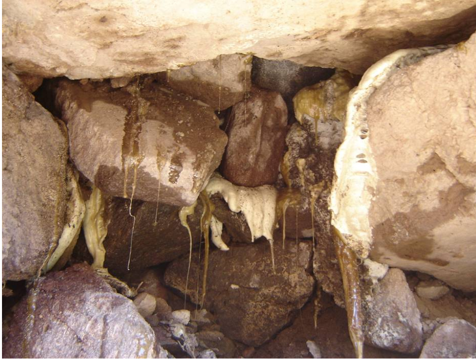
Figure 22. Photo. PUR product distribution within large void in dry-stack wall. This location was initially injected via jam-rods behind the wall the day after steady rains passed through the area, resulting in foaming of the PUR. Subsequent face injection days later, when the wall rock had dried substantially, resulted in non-foamed resin coverage of the interior rocks. The foamed PUR provides for consolidation, whereas the non-foamed product provides for rock-on-rock adhesion.
