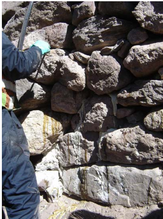
Figure 24. Photo. PUR injection directly between wall facing rocks using a hand-held injection nozzle.
