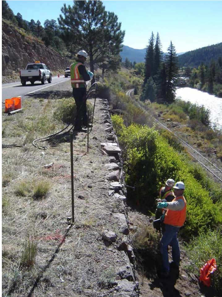
Figure 18. Photo. Jam-rods placed along the top of a well-built, well performing section of the study wall. No signs of wall settlement allowed placement of the injection rods closer to the wall face.
