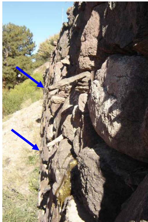
Figure 20. Photo. Blue arrows indicate location of balanced rocks used as “tell-tales” to detect outward wall deflection.
