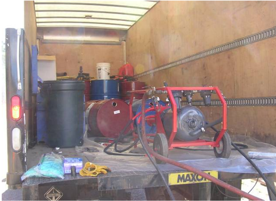
Figure 8. Photo. PUR Components A and B (red and blue barrels) and pumping system.
