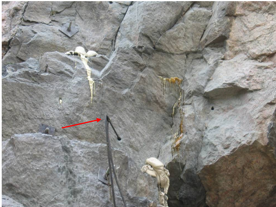
Figure 9. Photo. Migration of PUR from below the injection point # 11 (red arrow), upward through the rock mass. Note that some of the resin is foaming due to moisture in the surface fractures.
