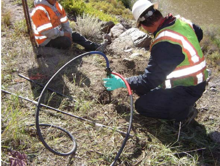
Figure 19. Photo. PUR A and B components are pumped separately to the top of the jam rod assembly. Mixing occurs within the injection rod assembly via a spiraled insert prior to product injection within the rock mass.
