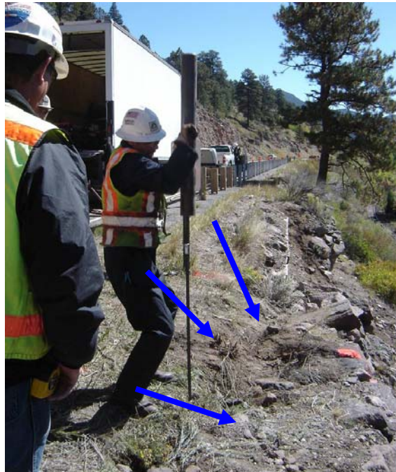
Figure 17. Photo. Driving jam-rod just behind visible wall settlement zone with fence post driver. Arrows indicate areas of wall displacement and settlement.
