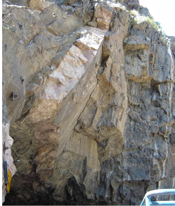
Figure 4. Photo. Close-up of the foliation joint-defined blocks above the western portal and previous spot-bolting.
