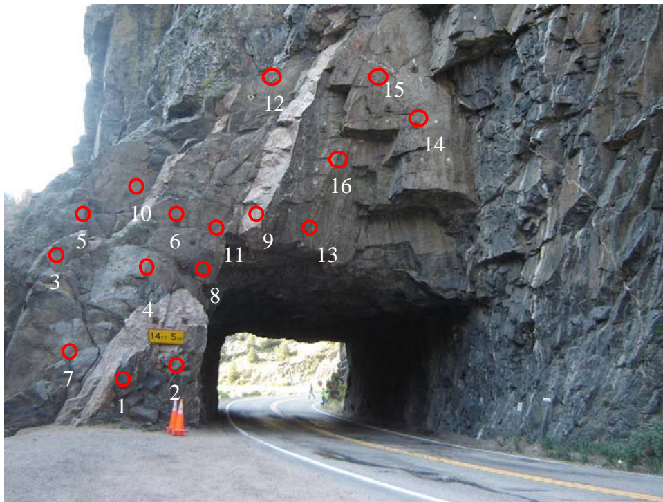
Figure 3. Photo. Western portal of the Poudre Canyon Tunnel with PUR injection hole sequence indicated in red (Approximate Locations).
