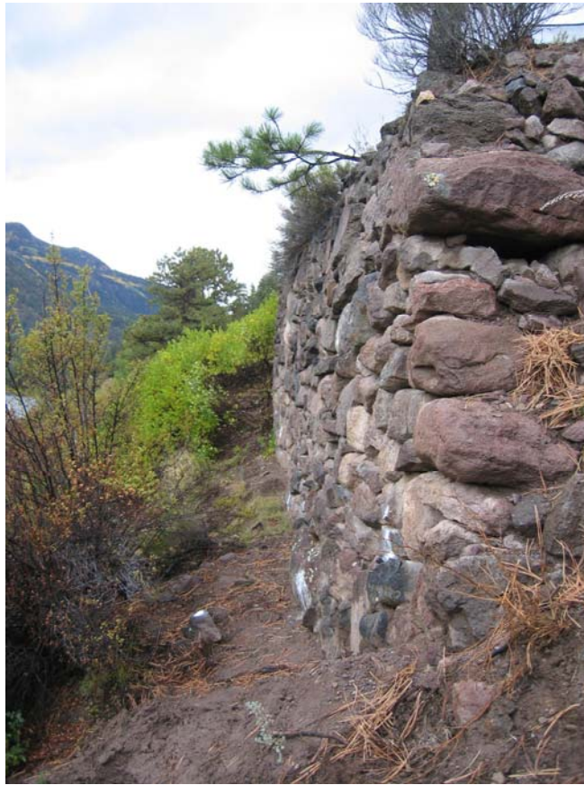
Figure 15. Photo. Bulging dry-stack wall, looking northwest along the test section.
