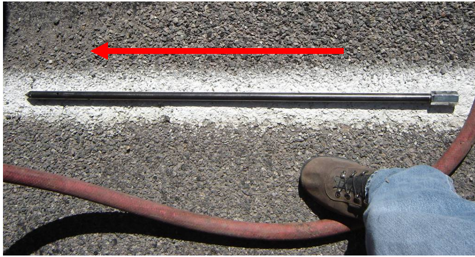
Figure 16. Photo. Jam-rod used to inject PUR product. Connection on right allows addition of extension rods, as needed. Injection ports are along the lower third of the jam-rod. Arrow indicates flow direction of product out of end port.
