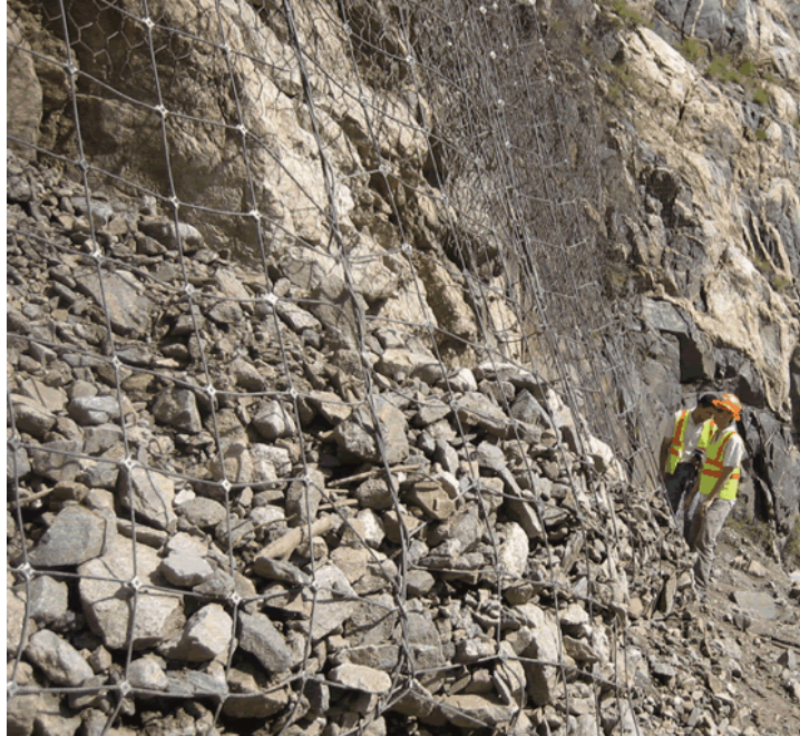
Figure 21. Photo. Rockfall Fence Containing an Overflow of Rock Fragments.
