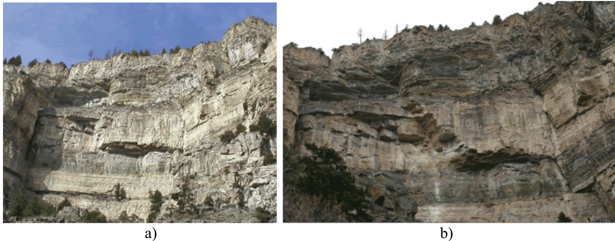
Figure 15. Photos. Section of Glenwood Canyon a) before, and b) after the 2004 Thanksgiving Day rockfall.
