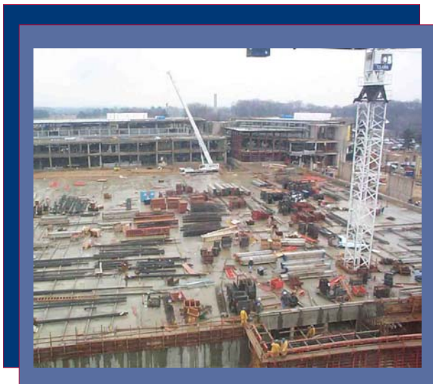
Construction is under way for a new laboratory at the National Institute of Standards and Technology in Gaithersburg, Maryland. Source: NIST
