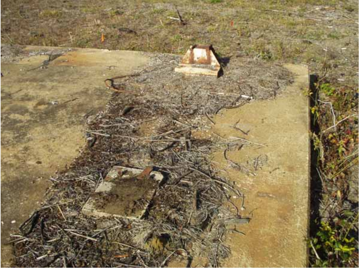
Details of item 28 looking NW at the north corner of the item.
