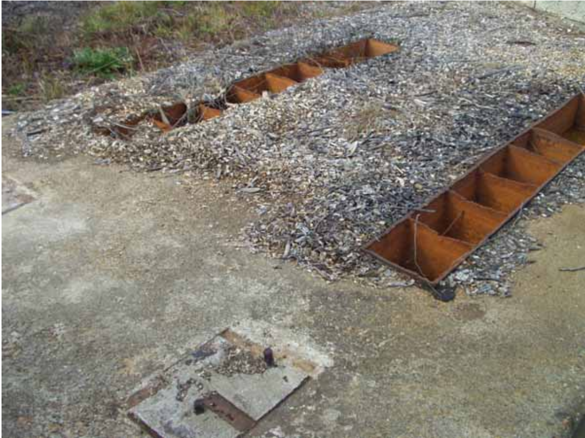
Detail of one of several similar areas of item 5.
