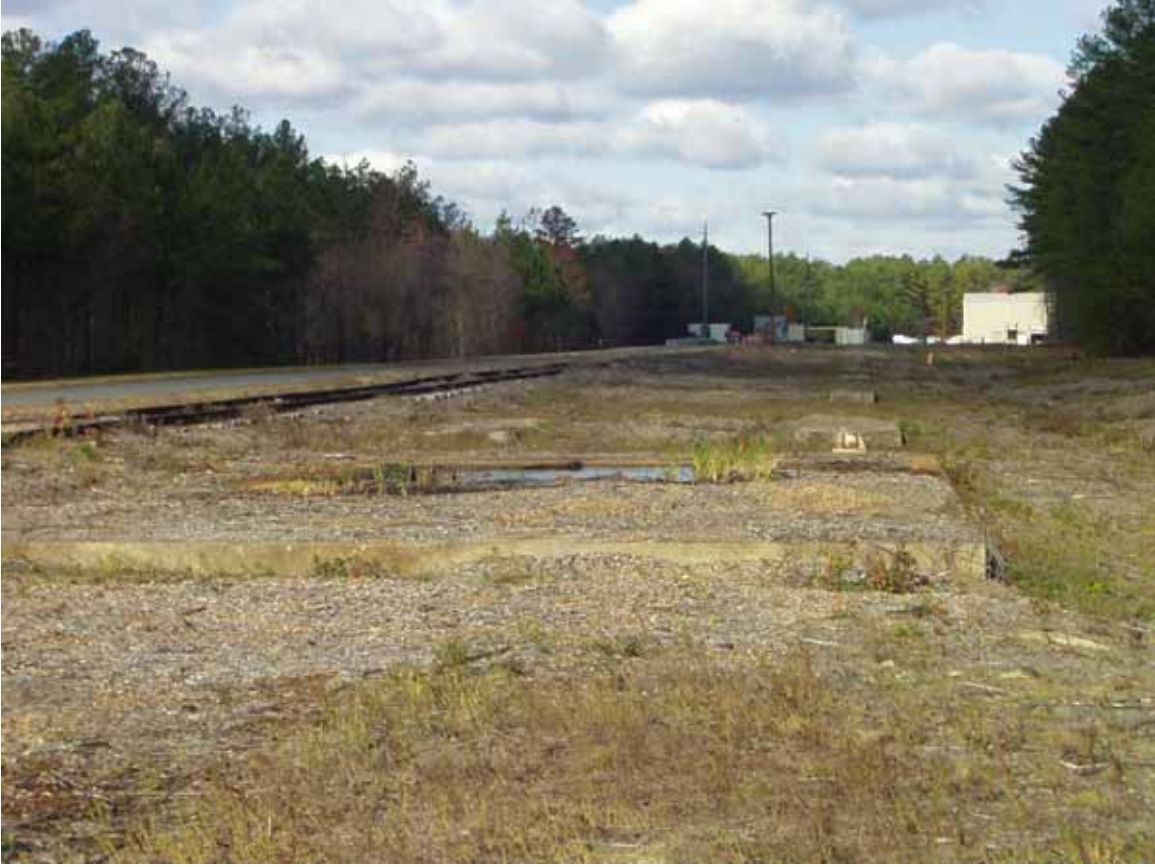
Looking NW at Item 28, note alignment with items 27 and other foundation pads in the background.
