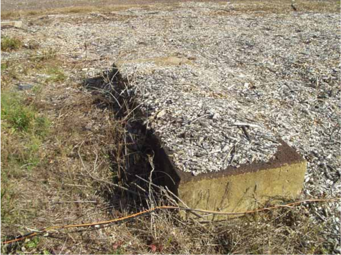
Item 2 First of three 3x9 items, looking NE. The Shock Tube foundation area is extensively covered with wood chips as a result of cutting and chipping of trees that had grown since the Shock Tube was in use. The wood chips are visible in nearly all pictures of the Shock Tube foundation.
