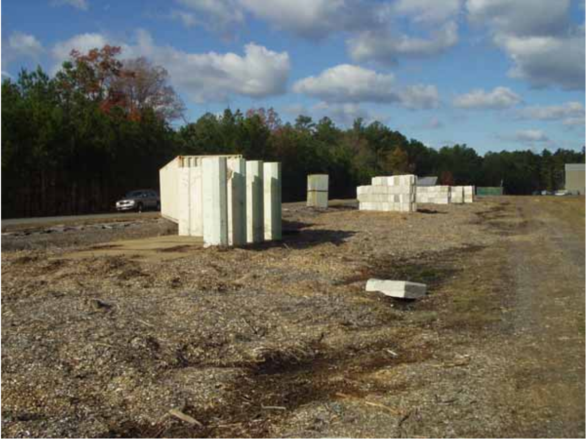
Looking northwest from item 8. Roof of building 1290A, green fence, and tan building 1410 are visible in the right background.
