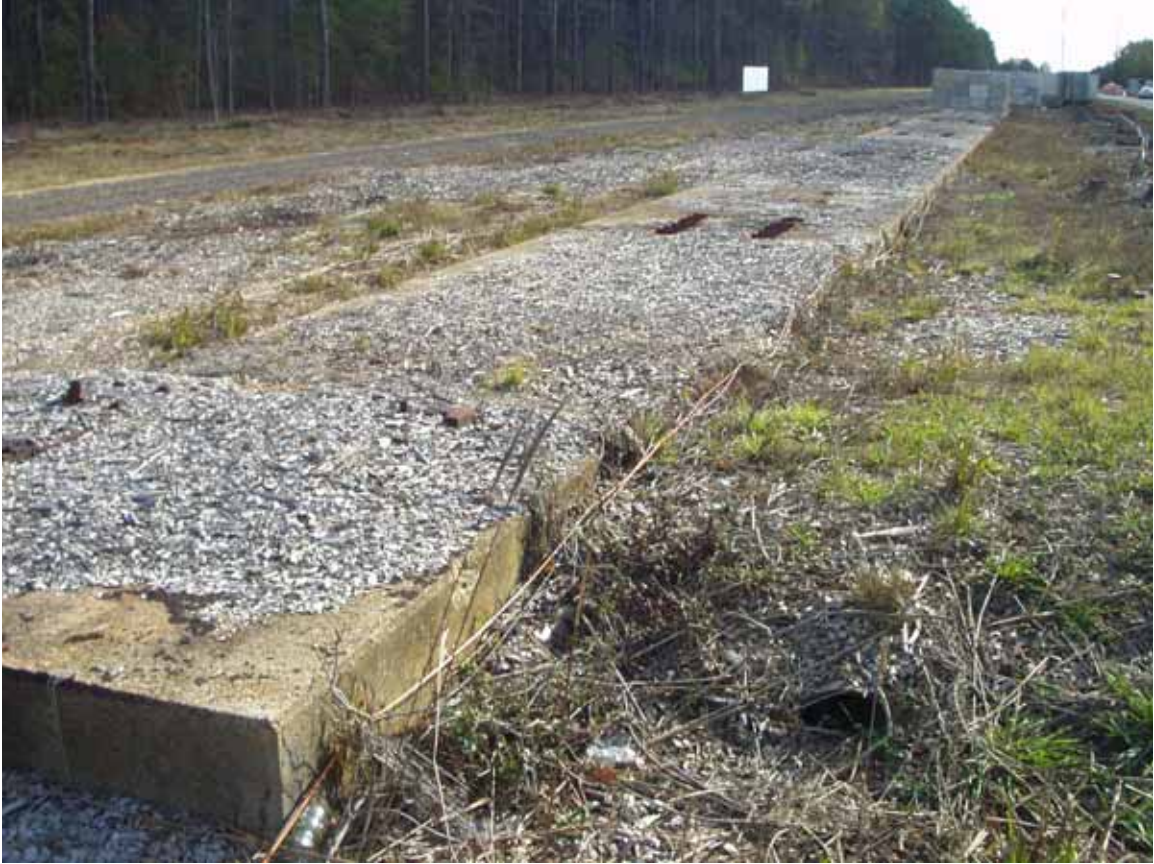
NW end of Item 5. Item 5 is approximately 10x230. One of two storm water pipes in what may be the remains of a railroad crossing in the right foreground.
