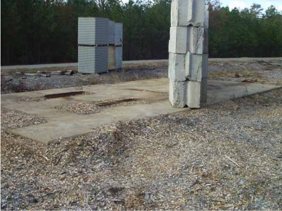
Item 7 looking west. Stacked gray blocks and the stacked corrugated boxes are not associated with the Shock Tube.
