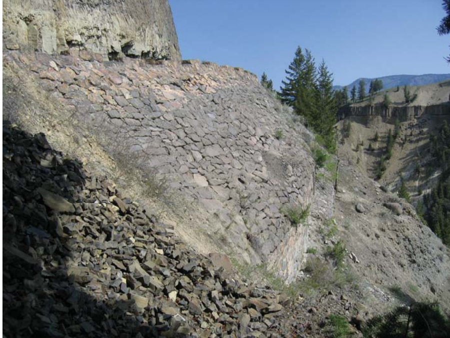
Figure 40. Photo. Dry-laid stone masonry wall at Yellowstone National Park built atop lower stone masonry wall (different construction periods?). The dimension, degree rock cutting, and placement quality of stone masonry work can vary greatly – even within a single wall.
