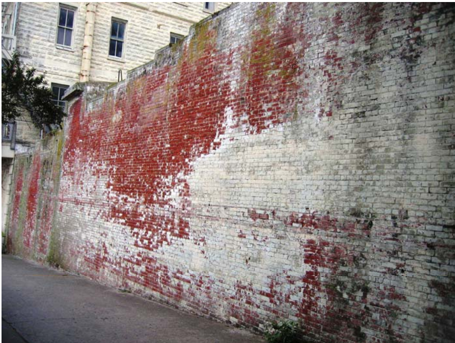
Figure 38. Photo. Tall painted brick wall at the Alcatraz unit of the Golden Gate National Recreation Area. Nearby concrete block walls suggest the interior of this wall may be constructed of larger blocks, with bricks added as a decorative facing.
