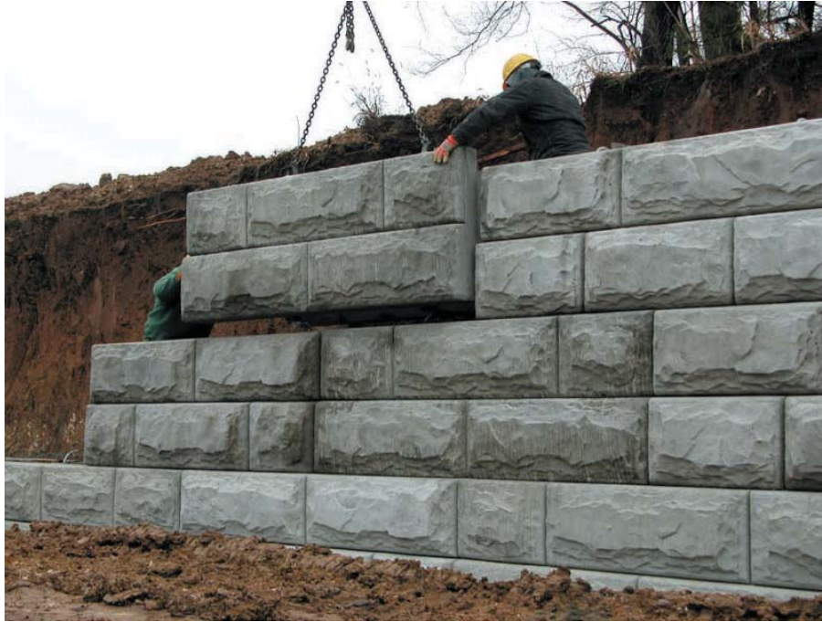
Figure 30. Photo. Precast hollow concrete “bin” blocks, with a formed architectural facing, are dry-laid at this cut wall installation and then aggregate filled for a rapidly-constructed, low-cost alternative to gravity concrete walls. (Courtesy Stone Strong, LLC)
