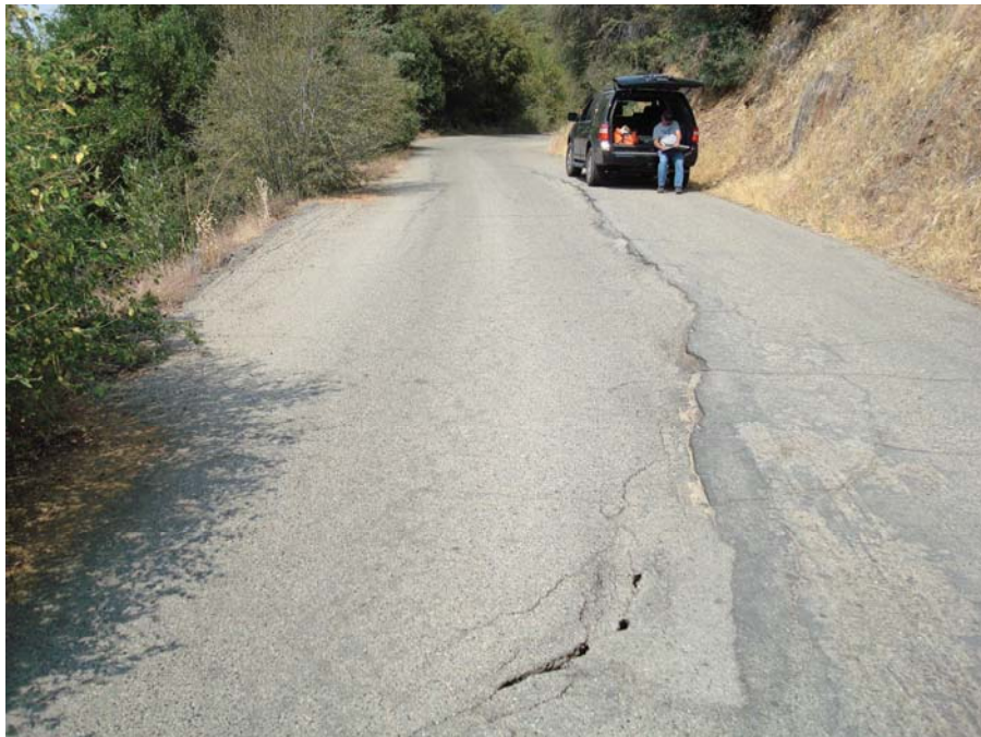
Figure 71. Photo. Severe roadway damage due to timber crib wall fill settlement, loss of fill material, foundation bearing failure or global slope instability (or combination thereof).
