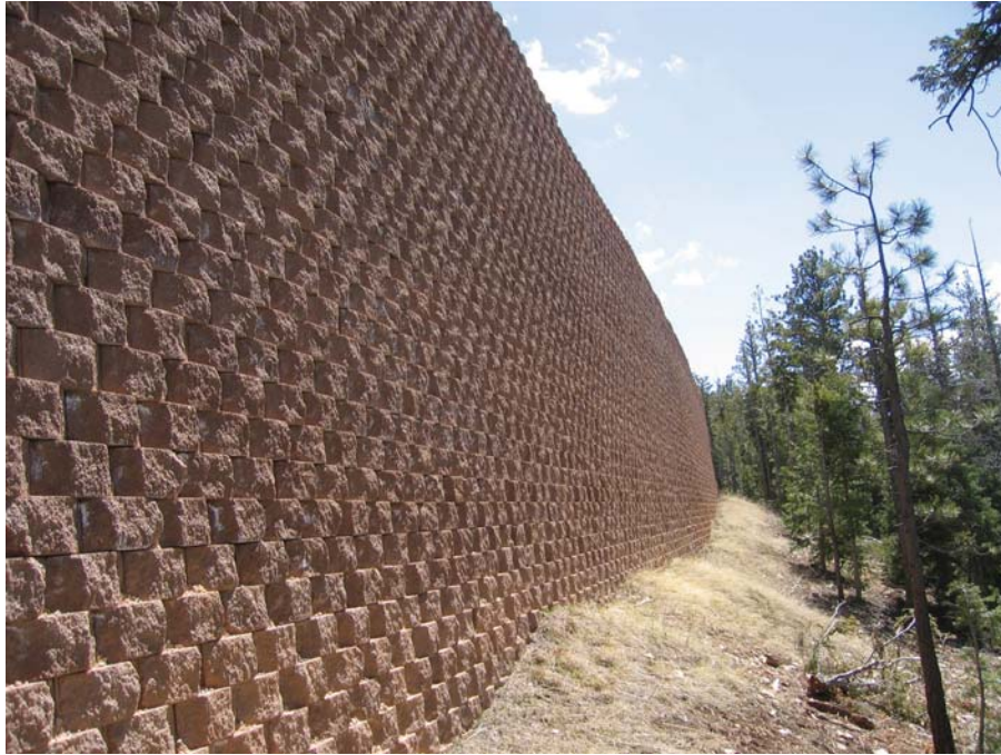
Figure 45. Photo. Segmental block wall with geogrid reinforcement at Bryce Canyon National Park. Although MSE walls can tolerate substantial settlements, brittle facings such as blocks or precast panels can result in severe cracking with relatively minor differential displacements.
