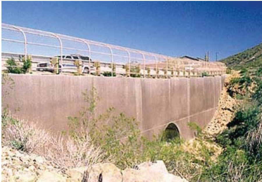
Figure 59. Photo. Example of float-finished, colored shotcrete applied over an MSE wall facing. (Courtesy Maricopa County, AZ)
