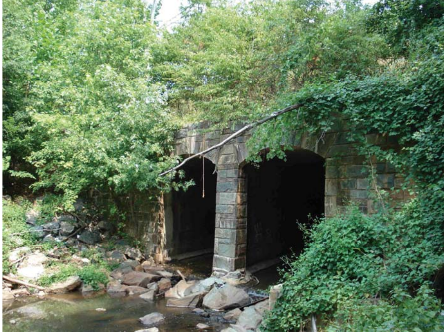
Figure 81. Photo. Culvert headwall along the Baltimore-Washington Parkway requiring removal of harmful vegetation along the top of the headwall. Vegetation removal was the most common type of maintenance item recommended throughout the Cycle 1 WIP inventory effort.
