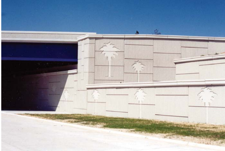
Figure 22. Photo. Example of secondary bridge walls (tiered MSE walls extending from the abutment and approach walls) that are not part of the bridge abutment structure and should be included in the WIP inventory.
