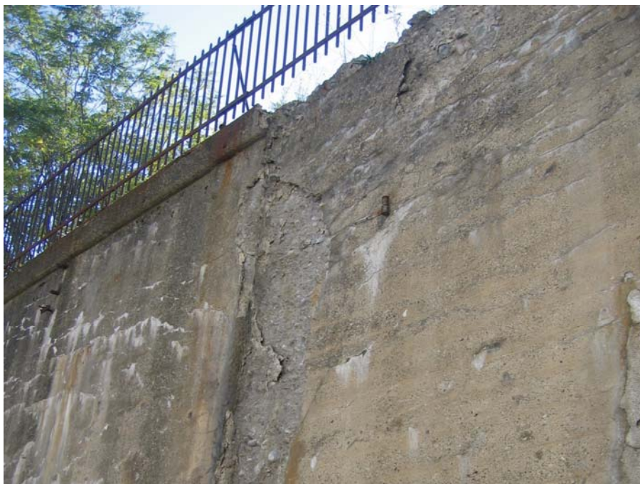
Figure 82. Photo. Much needed concrete repair on a cast-in-place gravity wall at Steamtown National Historic Site in Pennsylvania.
