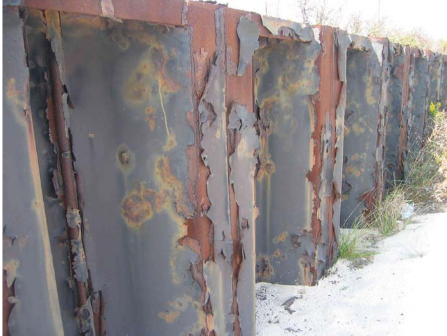
Figure 60. Photo. Severe weathering distress is evident on painted steel sheet piling at the Sandy Hook Unit, Gateway National Recreation Area. Less conspicuous weathering of painted surfaces can be difficult to discern without close inspection and knowledge of the most recent paint applications.
