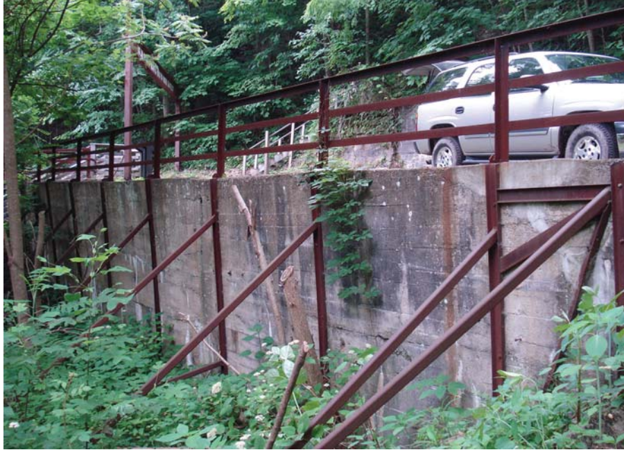
Figure 76. Photo. Developing wall problems at New River Gorge National River evidenced by post-construction remedial actions.
