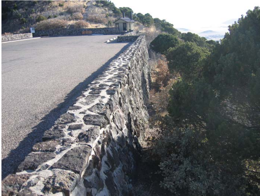
Figure 16. Photo. An example of parking area walls at Capulin Volcano National Monument. The wall in the foreground would be designated P1, the wall at the far end would be P2, and the wall partially shown on the left would be P3 per the WIP counterclockwise wall numbering notation for parking areas.
