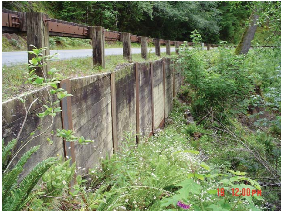
Figure 33. Photo. Timber-lagged, soldier pile fill wall employing steel H-piles at Olympic National Park. To limit wall deflection, unanchored soldier pile walls are generally restricted to heights well under 15 ft, depending on the size of piling employed. Both piles and lagging are commonly treated for corrosion and dry rot, respectively.
