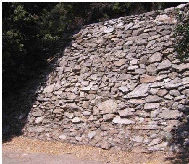
Figure 24. Photo. Example of a mortared stone masonry switchback wall at Sequoia National Park between upper and lower roadway on the inside of a switchback curve.
