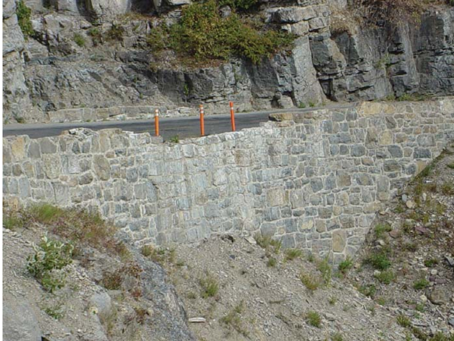
Figure 70. Photo. A section of parapet along this mortared stone masonry wall at Glacier National Park has been damaged due to vehicular impact. This portion of the wall would be assessed and rated under the “Traffic Barrier/Fence” secondary element.
