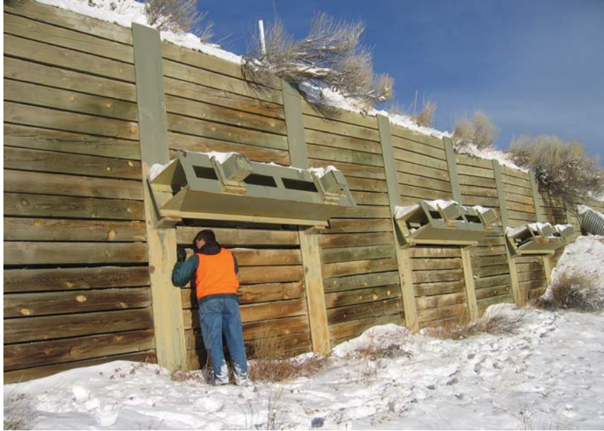
Figure 27. Photo. Timber-lagged soldier pile tieback wall at Mesa Verde National Park. A steel box-frame whaler assembly is used in this example as the bearing member for the ground anchors. Surface treatments are commonly applied to the timber lagging (weathering sealants) and exposed steel pile, whaler and ground anchor assemblies (paint).
