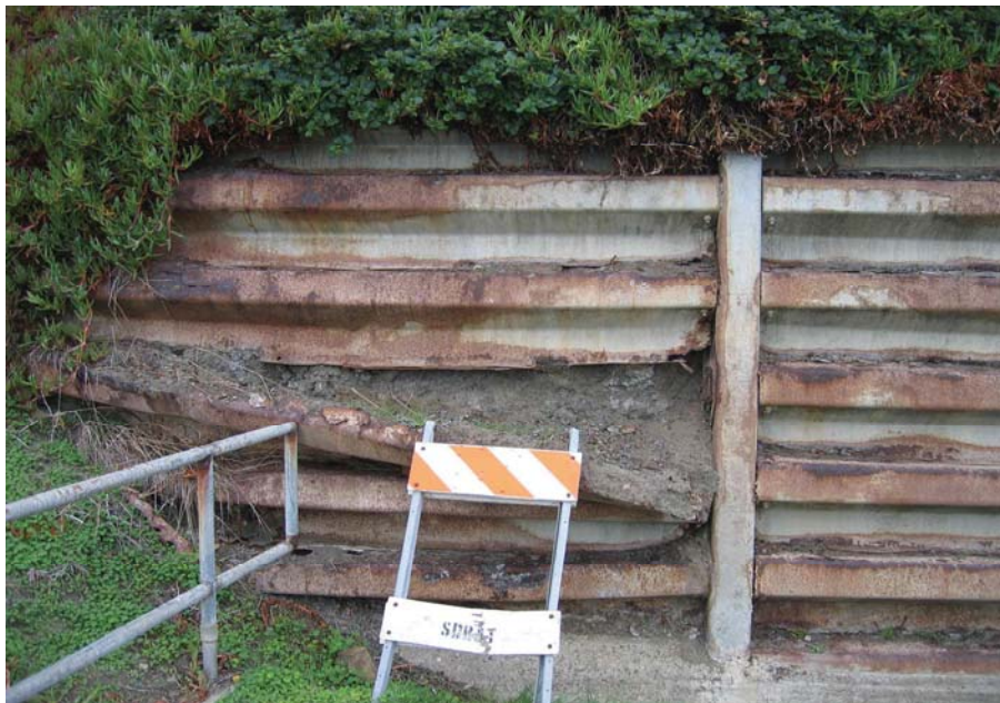
Figure 84. Photo. Severely corroded metal bin wall in serious need of complete replacement at China Beach within the Golden Gate National Recreation Area.
