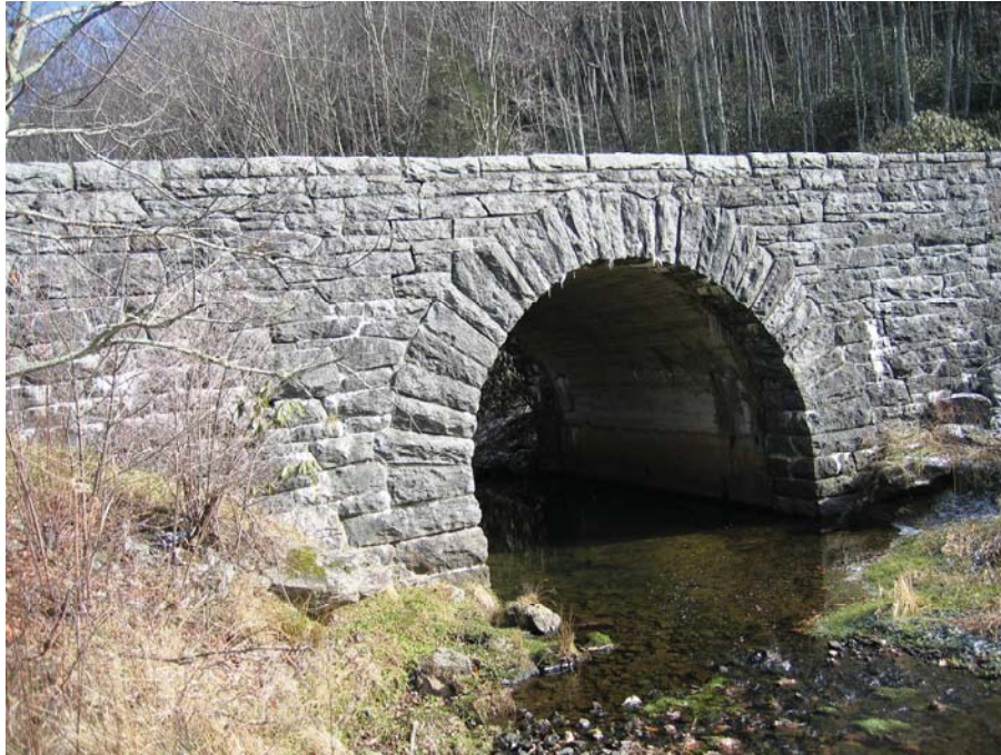
Figure 42. Photo. Mortared stone masonry head wall along the Blue Ridge Parkway. Although the mortar is often highly weathered in these structures, well-masoned and placed rock result in remarkably stable, high-performing, long-life structures.
