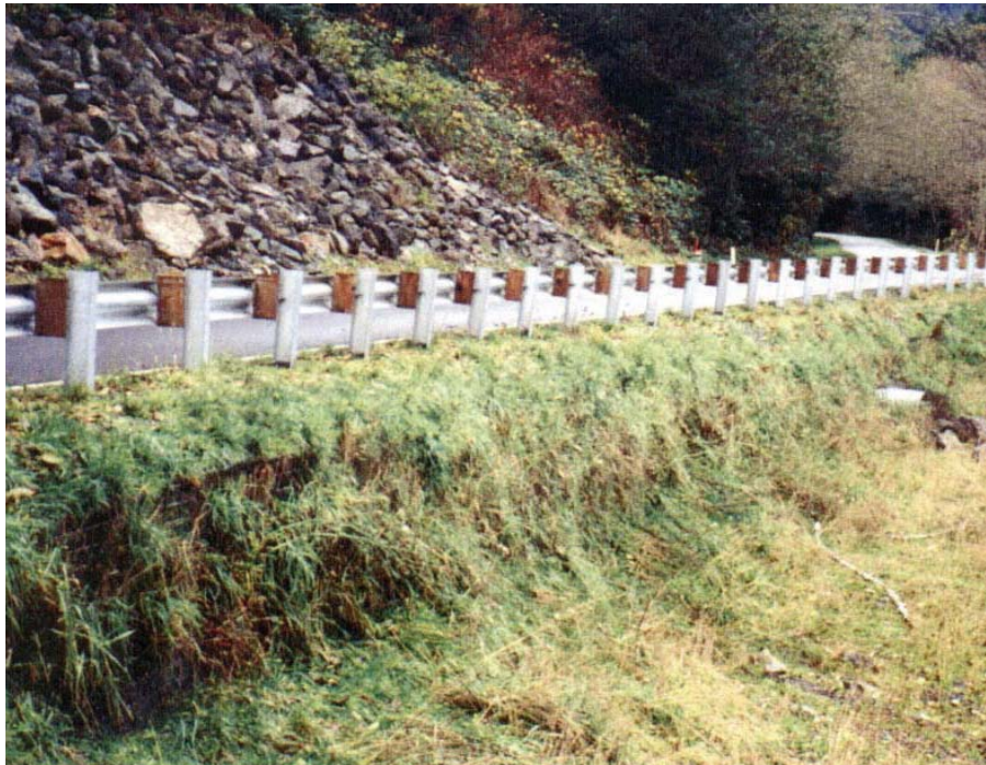
Figure 53. Photo. A well-vegetated wire-faced MSE wall in Siskiyou National Forest. Grasses, small bushes and other forms of light ground cover are appropriate for vegetated wall faces. Trees growing from the wall face or along the top of the wall, present a wall performance threat.
