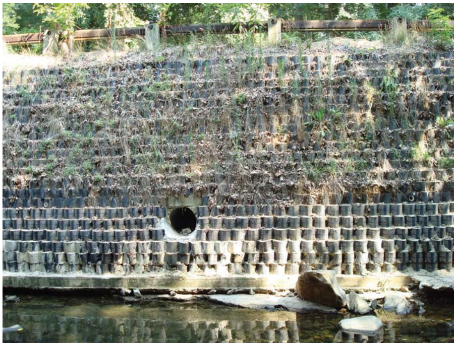
Figure 49. Photo. “Other” wall type: geosynthetic reinforced earth wall with planted geocell facing. This wall facing method may prove to be a superior means for establishing face vegetation in high growth climates. Note the installation of the concrete leveling pad.
