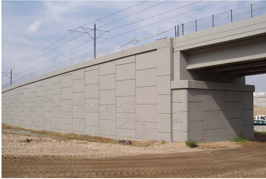
Figure 20. Photo. Although the approach walls are integral to the bridge abutment, they extend sufficiently from the end of the deck to be considered fill walls primarily supporting the roadway. Approach walls such as these should be included in the WIP inventory if not already evaluated under the BIP program.
