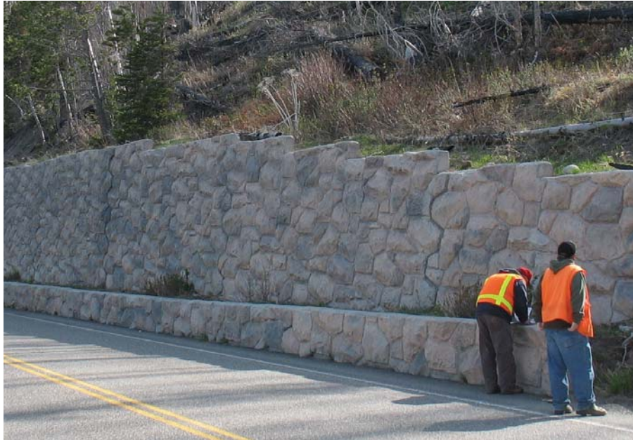
Figure 47. Photo. Soil nail wall at Yellowstone National Park with a form-lined, cast-in-place simulated stone structural facing. The formliner is subsequently stained or painted to better simulate natural stone.
