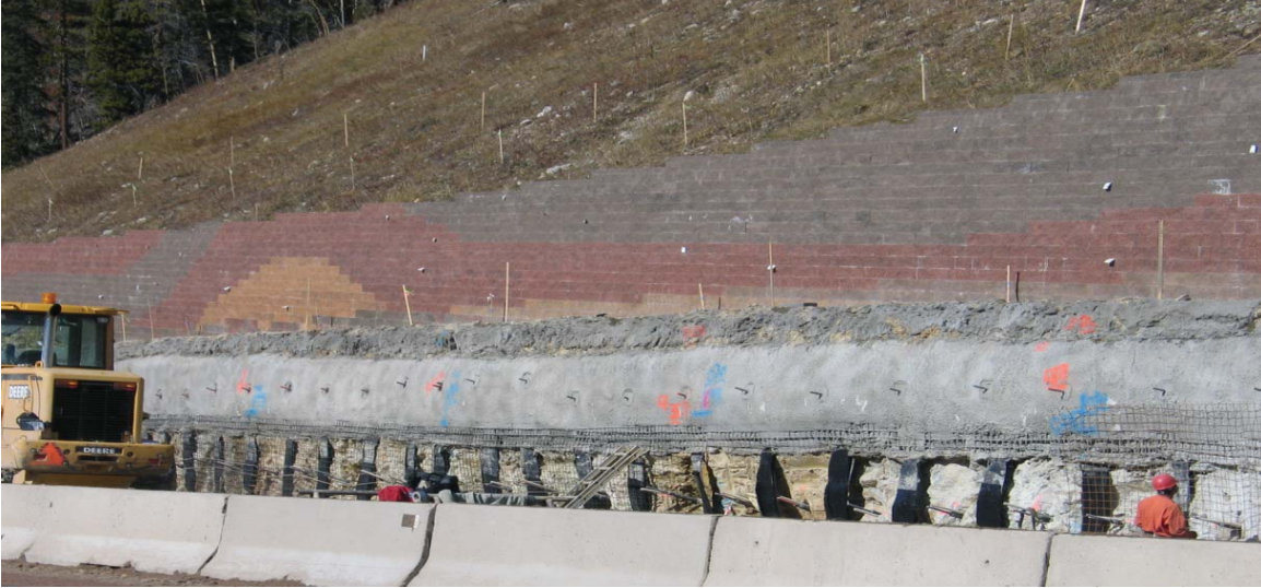
Figure 6. Photo. Multi-tiered soil nail wall under construction with decorative modular block facing. Without input from knowledgeable park staff, the wall inventory might overlook the soil nail reinforcing elements when evaluating the completed structure.
