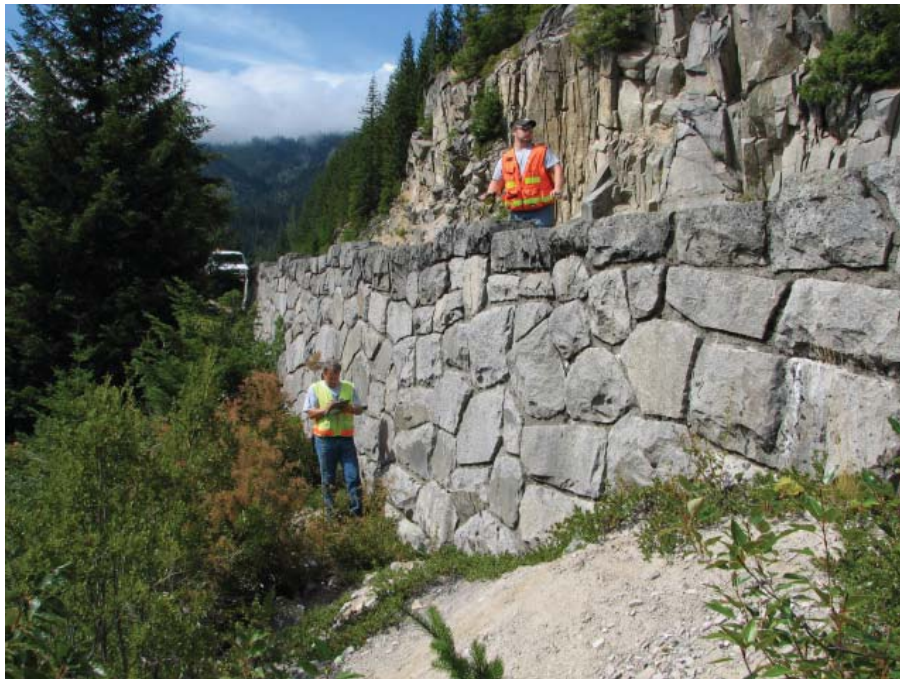
Figure 1. Photo. Two-man inventory team measures and assesses the condition of a mortared stone masonry gravity fill wall, with integral guardwall parapet, at Mount Rainier National Park.
