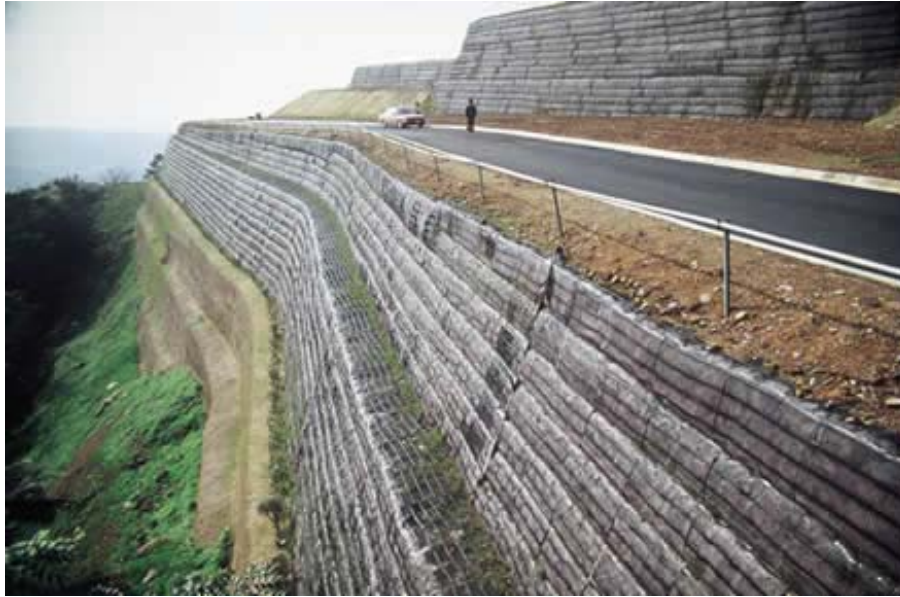
Figure 43. Photo. Multi-tiered, plantable, geosynthetic wrapped MSE wall. Although UV-resistant materials are available, the inspecting engineer should pay close attention to the degradation of exposed geosynthetics versus the age of the wall. (Courtesy Tensar Corp.)
