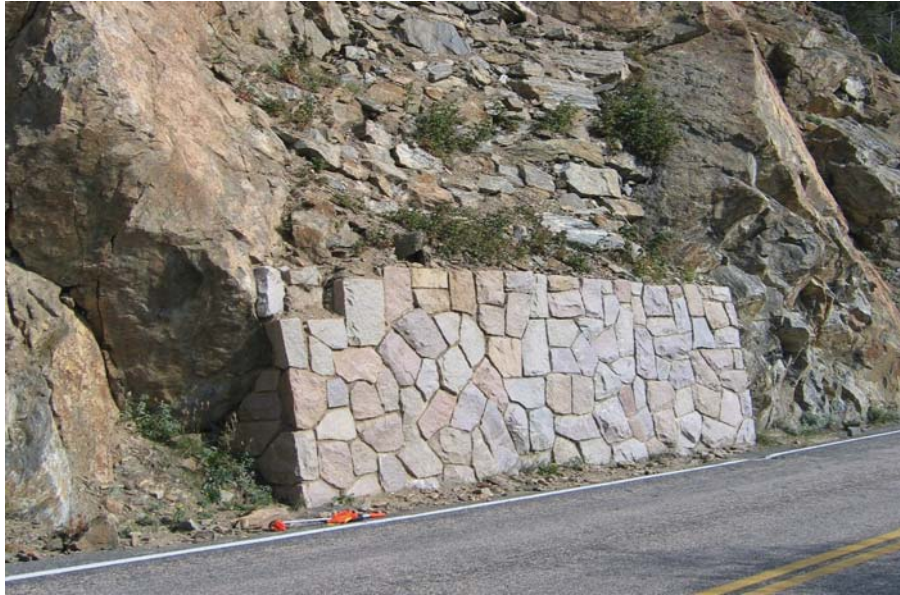
Figure 18. Photo. A mortared stone masonry cut wall at Rocky Mountain National Park.
