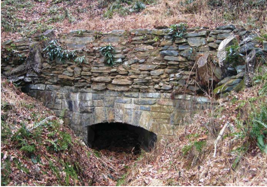
Figure 67. Photo. A mortared stone masonry headwall along the Blue Ridge Parkway, subsequently overlain with a dry-laid, placed-stone retaining wall built around trees growing at either end of the headwall.
