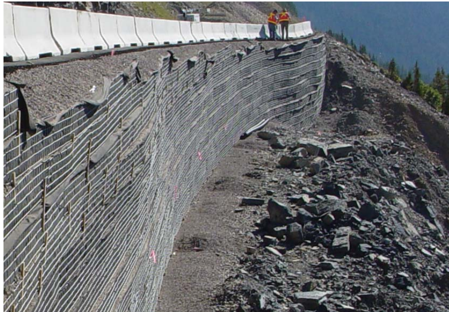
Figure 73. Photo. MSE wall at Glacier National Park awaiting final facing. The bench in front of the wall would be evaluated as a “Wall Foundation Material” primary element. The rocky slope below the bench would be evaluated as a secondary element under “Downslope”.
