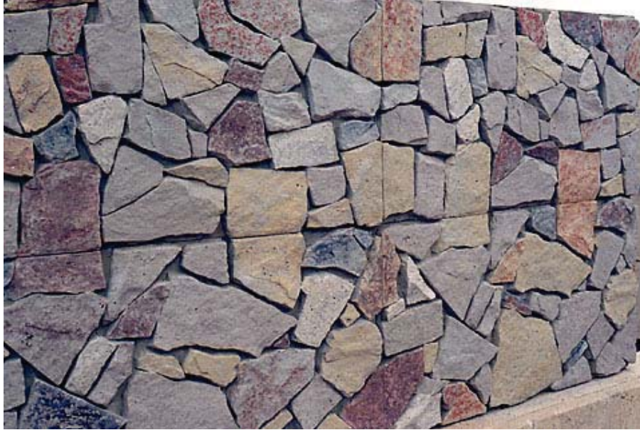
Figure 56. Photo. Simulated stone using a deep-inset formliner and individually stained rock units. This application attempted to disguise the form joints by matching whole rocks panel-to-panel. (Courtesy Vail Associates)
