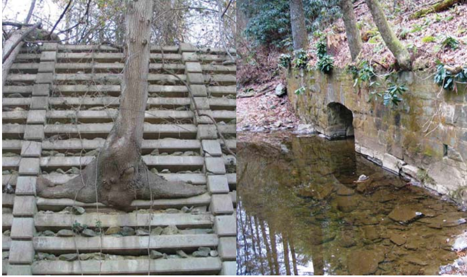
Figure 74. Photo. Left unchecked, trees will grow just about anywhere, and can cause severe damage to retaining walls.
