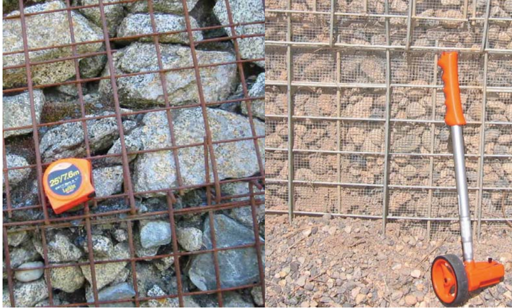
Figure 64. Photo. Not all MSE wall facing systems are the same. Mats may or may not be galvanized (left) and, depending on the size of facing fill versus the minimum wire mat opening, hardware cloth may or may not be required for fill retention (right).
