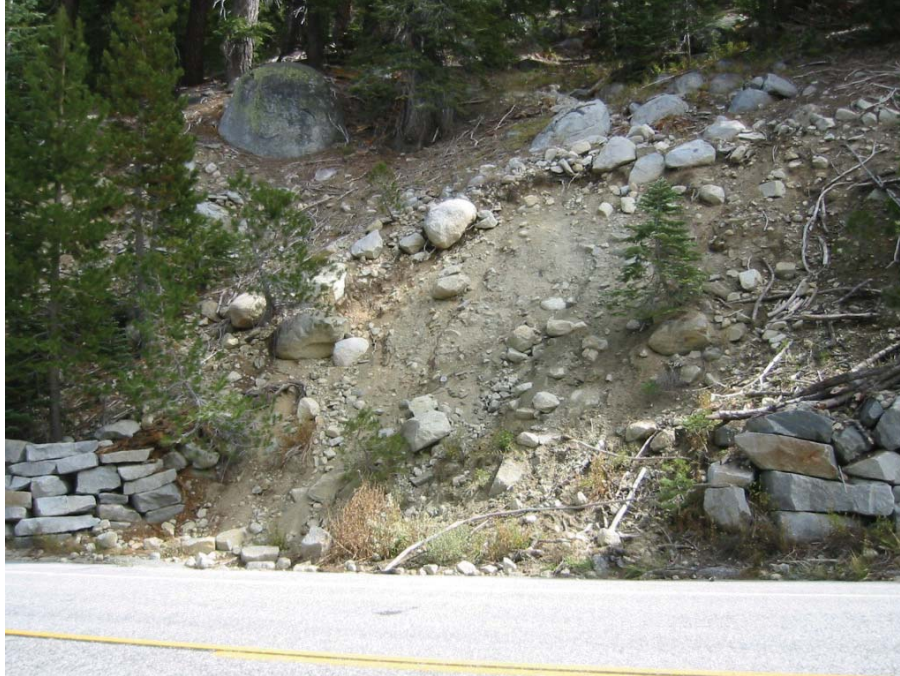
Figure 83. Photo. Dry-laid stone masonry elements in need of replacement at Yosemite National Park following minor slope instability.
