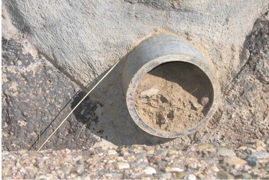
Figure 69. Photo. Plugged “weephole” drain at bottom of mortared stone masonry wall.
