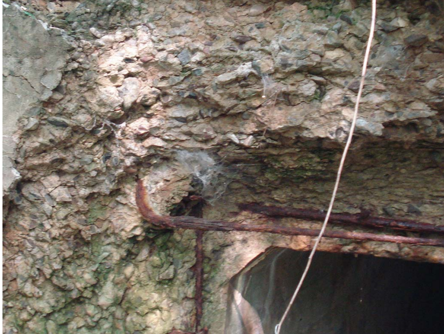
Figure 65. Photo. Severely weathered reinforced concrete headwall at Delaware Water Gap National Recreation Area.
