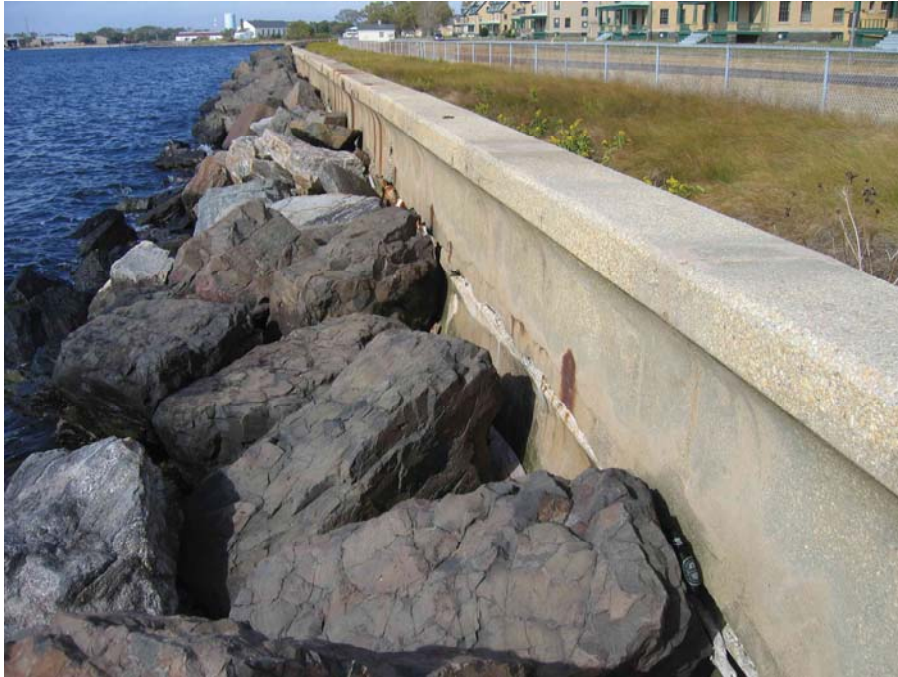
Figure 25. Photo. Although this seawall at the Sandy Hook unit of the Gateway National Recreation Area sits well outside the construction limits of the RIP-surveyed road (back right), failure of this structure would result in rapid and severe shoreline erosion, eventually impacting the roadway.
