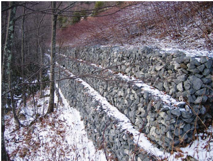
Figure 41. Photo. Angular rock fill gabion wall at the toe of a large fill along the Blue Ridge Parkway.
