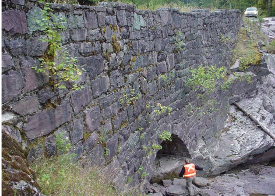
Figure 23. Photo. Is it a fill wall with an elaborate culvert structure, or a culvert with an elaborate headwall? In this case, the outlet was considered a large retaining wall with a culvert, whereas the much smaller inlet was considered a culvert headwall.
