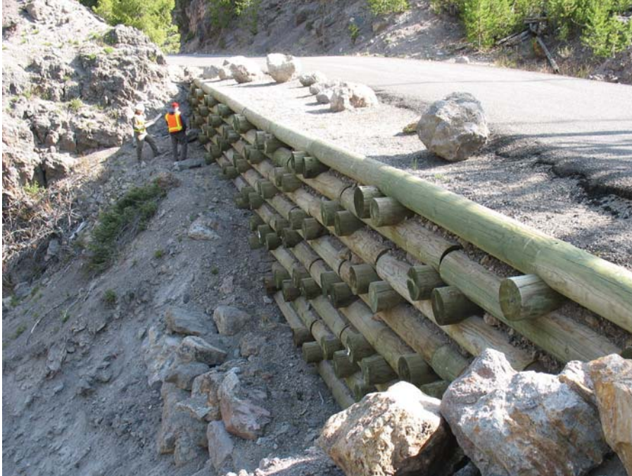
Figure 37. Photo. Timber crib wall at Yellowstone National Park employing large-diameter logs set “Lincoln Log” style on a placed rock fill.
