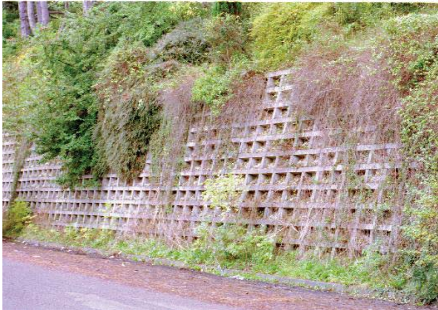
Figure 78. Photo. A sizeable portion of this concrete crib wall is obscured by heavy vegetation. Although observed conditions are sufficient to rate the condition of wall elements, additional investigations might be required or recommended to better understand element performance, particularly if material or structural problems were suspected. (Data Reliability Factor = 2)
