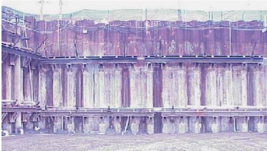
Figure 29. Photo. Steel sheet piling with bar ground anchors placed through steel whalers. This cut wall is constructed “top-down”, with the ground in front of the driven sheet piles excavated in lifts and ground anchor assemblies installed as the excavation proceeds to final grade.
