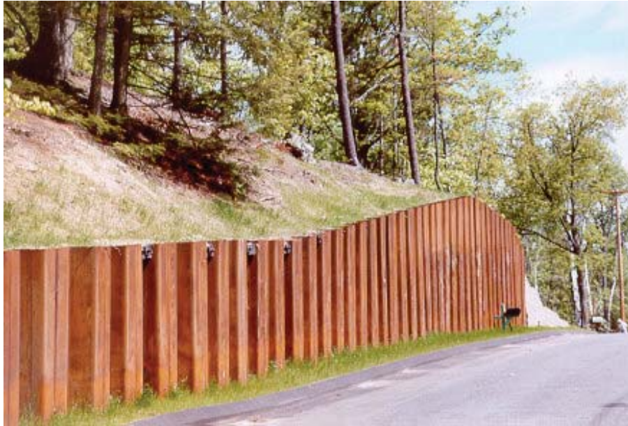
Figure 34. Photo. Cantilever steel sheet pile cut wall with “deadman” anchors placed at the top of the wall to support the higher wall sections.
