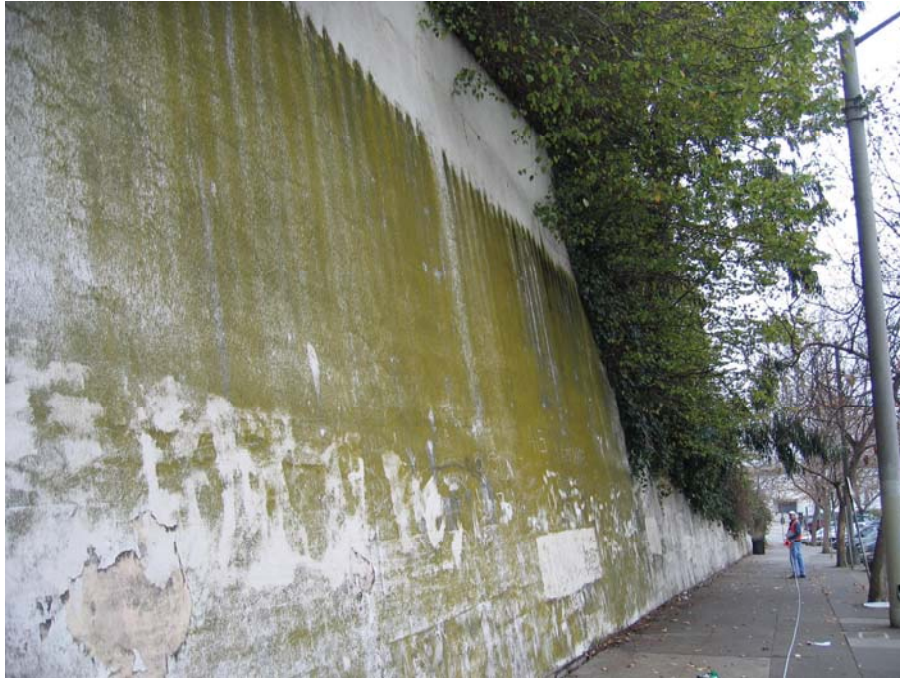
Figure 39. Photo. Painted mass concrete gravity wall bordering Ft. Mason at the Golden Gate National Recreation Area. Although less aesthetically appealing than other wall types or facings, the inspecting engineer should nonetheless be aware of the cultural sensitivity of these structures.
