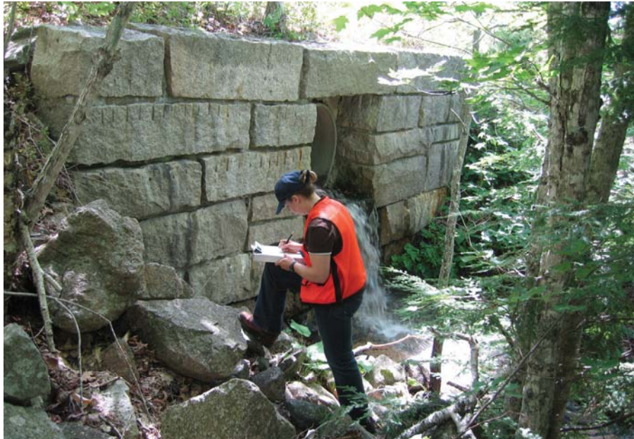
Figure 2. Photo. Assessment of a culturally significant culvert headwall at Acadia National Park.
