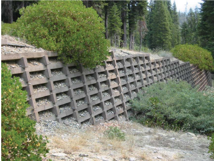
Figure 35. Photo. Concrete crib wall at Sequoia National Park. This wall is filled with crushed aggregate, though many similar structures may be constructed with planted faces.
