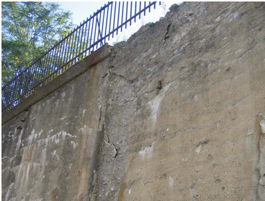
Figure 82. Photo. Much needed concrete repair on a cast-in-place gravity wall at Steamtown National Historic Site in Pennsylvania.
