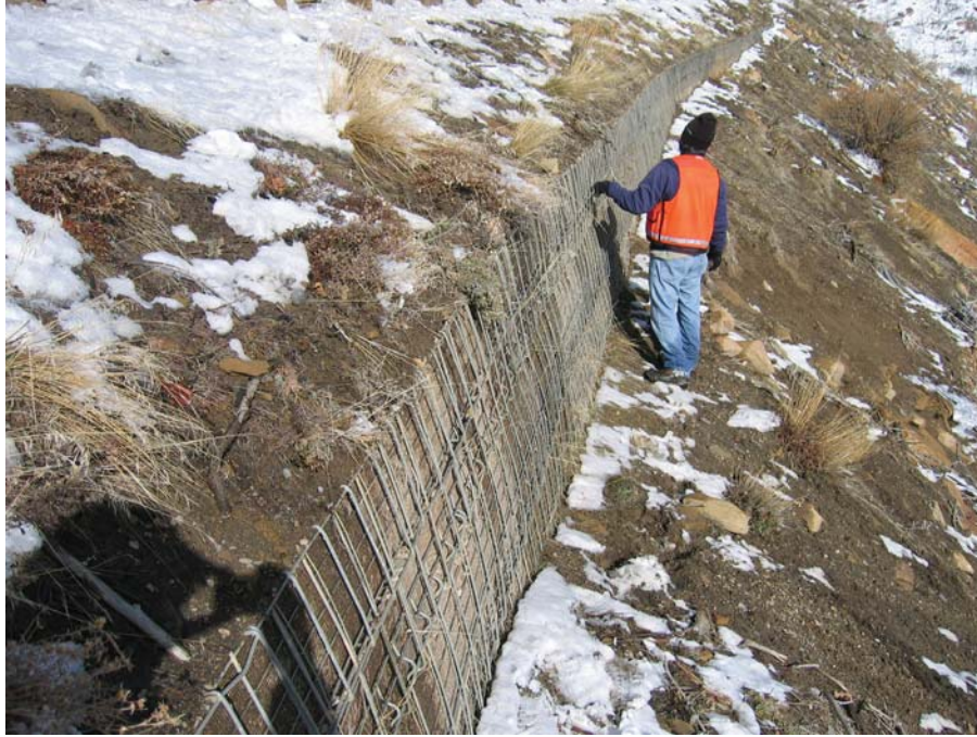
Figure 14. Photo. A mid-slope wire-faced MSE wall at Mesa Verde National Park that just meets the height criterion based on known embedment of partially-exposed lower baskets.
