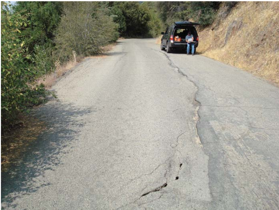
Figure 71. Photo. Severe roadway damage due to timber crib wall fill settlement, loss of fill material, foundation bearing failure or global slope instability (or combination thereof).
