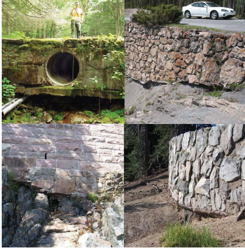
Figure 68. Photo. Examples of deteriorating wall foundation conditions: (clockwise from upper left) outlet scour at culvert headwall, Great Smoky National Park; soft soil erosion from under mortared stone masonry walls at Yellowstone and Crater Lake National Parks; deteriorating rock foundation at Acadia National Park.
