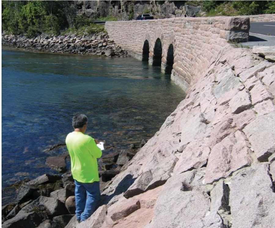
Figure 19. Photo. Example of a highly battered, dry-laid stone masonry wall supporting the bridge approach at Acadia National Park. This wall is not integral to the bridge structure and, therefore, should be assessed as a retaining wall under the Wall Inventory Program.
