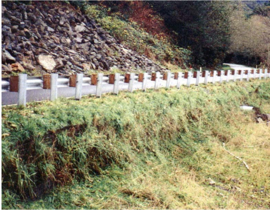
Figure 53. Photo. A well-vegetated wire-faced MSE wall in Siskiyou National Forest. Grasses, small bushes and other forms of light ground cover are appropriate for vegetated wall faces. Trees growing from the wall face or along the top of the wall, present a wall performance threat.
