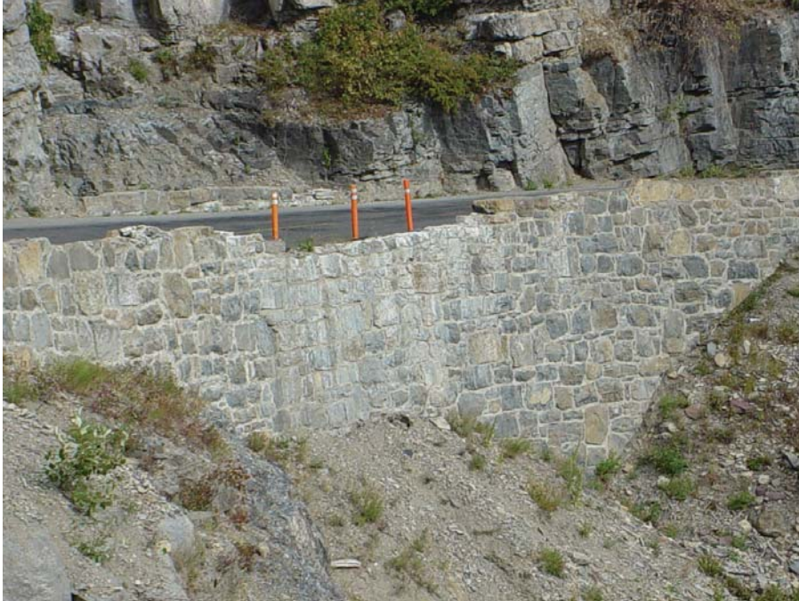
Figure 70. Photo. A section of parapet along this mortared stone masonry wall at Glacier National Park has been damaged due to vehicular impact. This portion of the wall would be assessed and rated under the “Traffic Barrier/Fence” secondary element.
