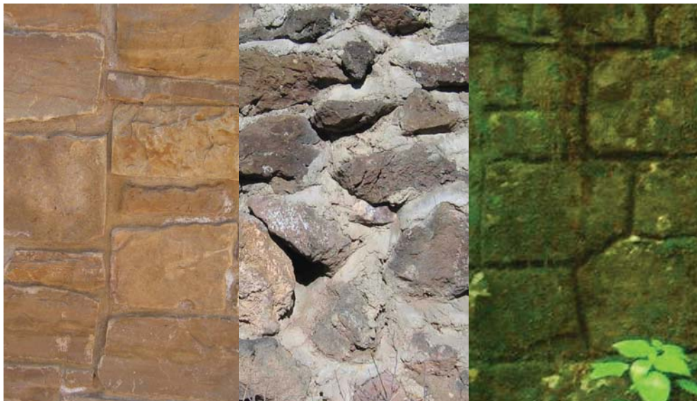
Figure 66. Photo. Not all mortar applications are the same: (from left-to-right) highly-crafted mortar placement on fairly new wall at Bryce Canyon National Park; poor, inconsistent mortaring at Capulin Volcano National Monument; well-placed, yet highly weathered mortar showing signs of excessive seepage through headwall at Great Smoky Mountains National Park.
