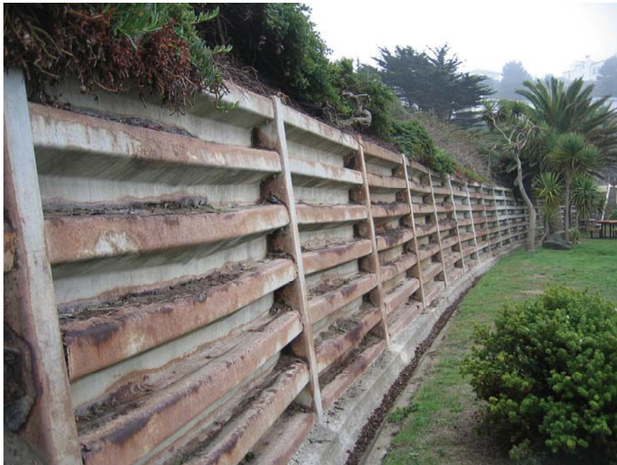
Figure 31. Photo. Heavily corroded metal bin wall at China Beach, Golden Gate National Recreation Area. Constructed in the 60’s, the protective coating on the exposed bin facing elements has long since deteriorated.
