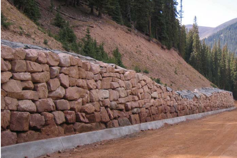
Figure 79. Photo. Although built to strict material and construction standards, this new rockery wall along the Guanella Pass Road in Colorado is a non-AASHTO design.
