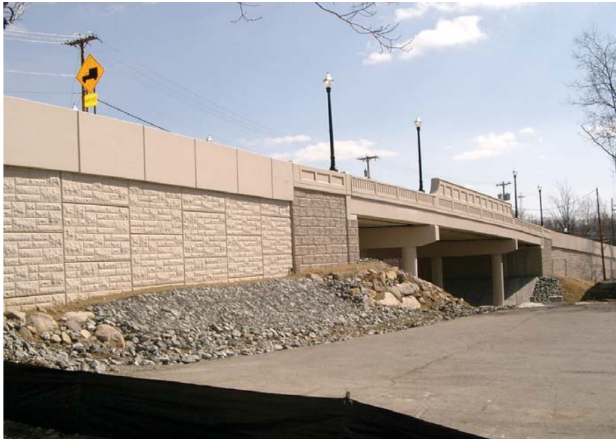
Figure 21. Photo. Example of approach walls clearly distinguished from the bridge abutment by a constructive joint, approximately 15 feet from the end of the deck.
