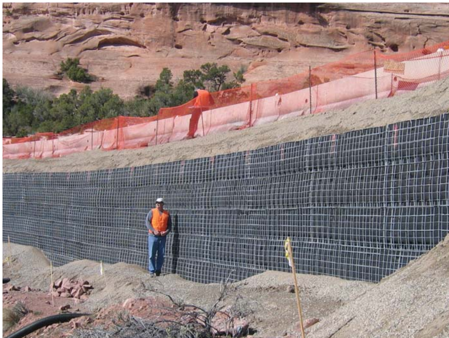
Figure 46. Photo. Wire-faced MSE wall, nearing completion at Colorado National Monument, utilizes a geosynthetic fabric to ensure retention of the metallic-grid reinforced aggregate. Left unprotected, this facing system would be susceptible to UV damage in the years to come.
