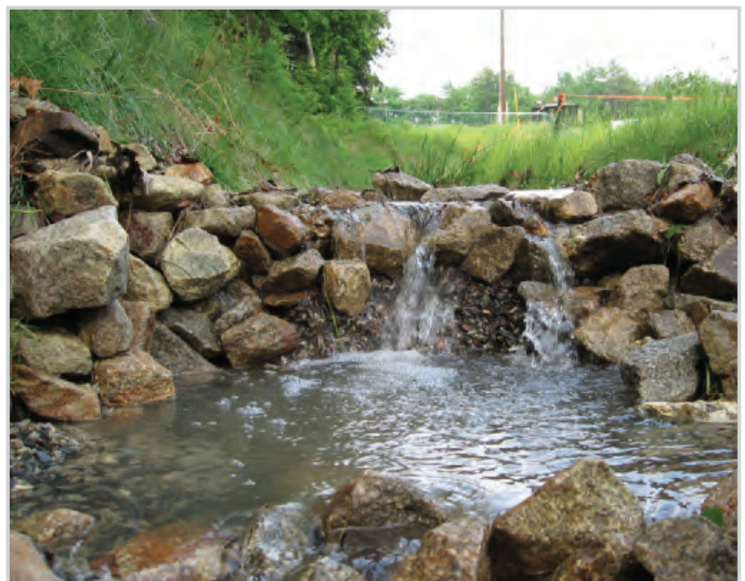
In April 2007 the filter berm swale failed after a torrential storm in which the swale conveyed a 6.8 cfs peak flow (more than six times the design flow).
