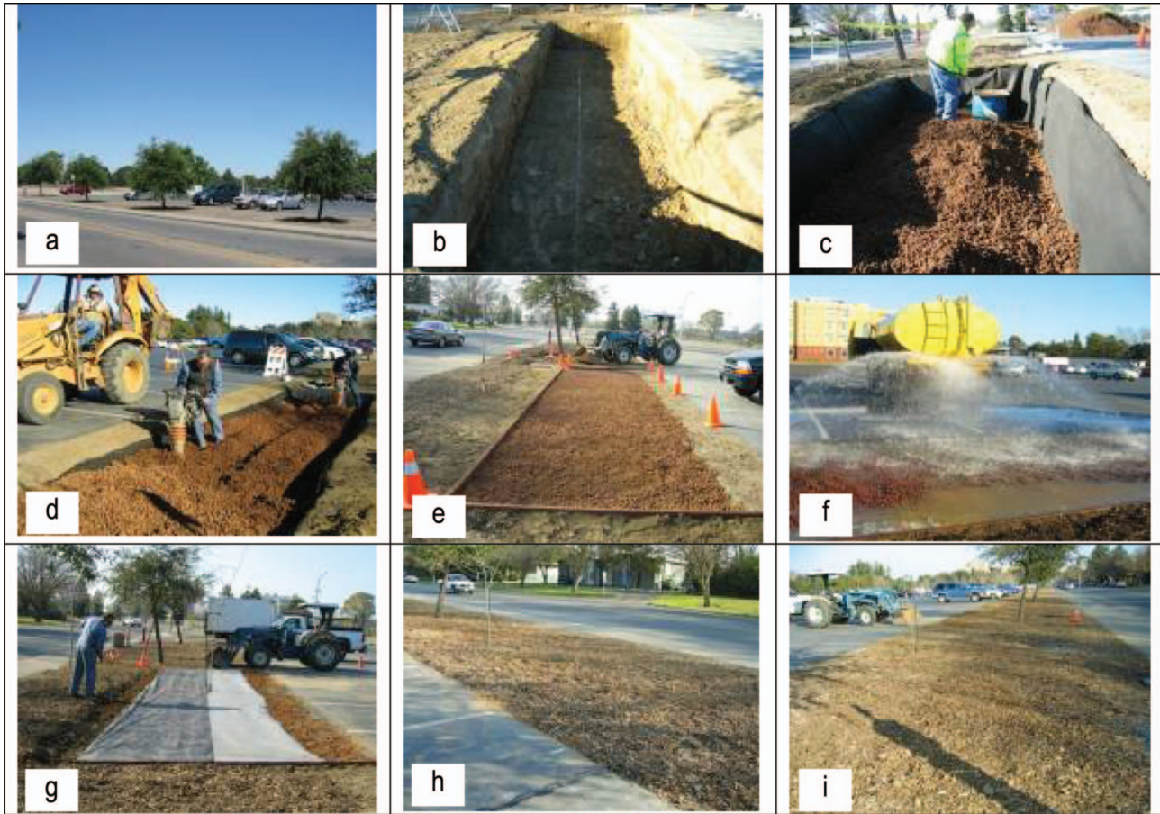
Figure 3. Field installation. Photos were taken at different stage of the field installation. a) Before the bioswale installation, b) excavated pit, c) filled with engineered soil, d) compacted the soil, e) leveled the pit, f) tested the soil settlement, g) added tree to the system, h) finished site, i) both control and treatment sites were covered with mulch to match the surrounding land cover.
