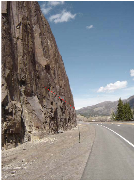
Figure 58. Photo. A rockfall-prone slope draped with unsecured wire mesh. Wolf Creek Pass, Colorado.
