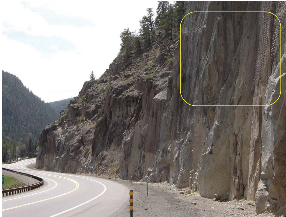
Figure 60. Photo. Rock slope treated with colored draped rockfall mesh.
