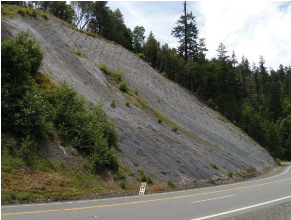
Figure 62. Photo. An anchored Tecco mesh system secured by a grid of rock bolts, US 299 in Northern California.
