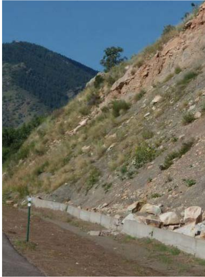
Figure 67. Photo. Concrete barriers used as a rockfall protection measure. Notice the damage caused by a large rock impact.
