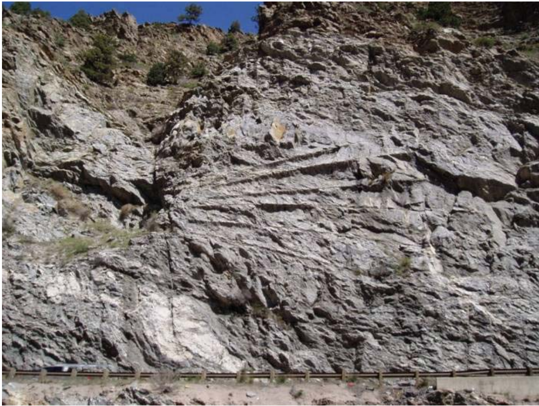
Figure 17. Photo. Drill hole traces left by horizontal drilling parallel to the rock face (fan drilling).
