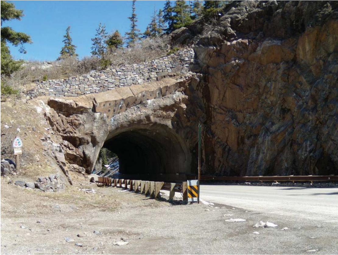
Figure 52. Photo. Sculpted shotcrete used to stabilize a tunnel portal (the area directly below the dry-stack wall is the sculpted shotcrete).
