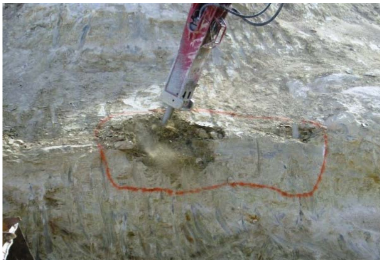
Figure 24. Photo. A hydraulic hammer sculpting a rock face (the material to be removed has been outlined with common marking paint).
