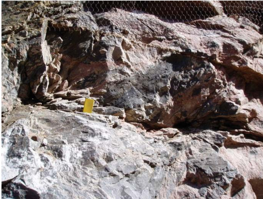
Figure 18. Photo. Blast damage caused by horizontal drilling perpendicular to the rock face.
