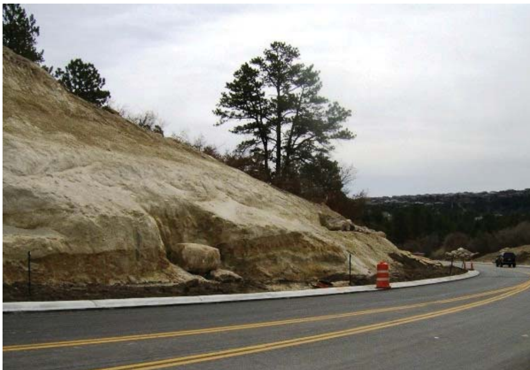
Figure 26. Photo. Completed rock slope prior to placement of topsoil and a native seed mix.
