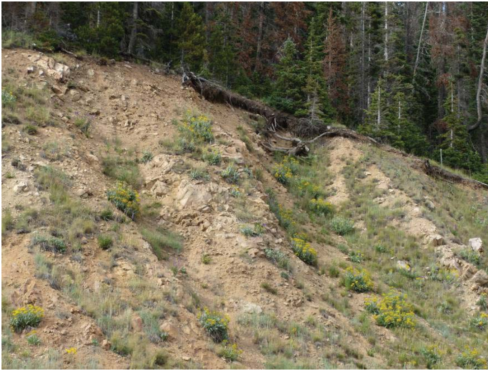
Figure 29. Photo. Expanded slope rounding can prevent this type of erosion and overhang.
