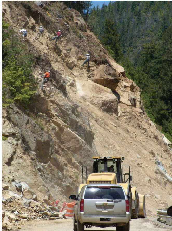
Figure 39. Photo. Hand scalers removing loose material from a cut slope South Fork Smith River Road, California.
