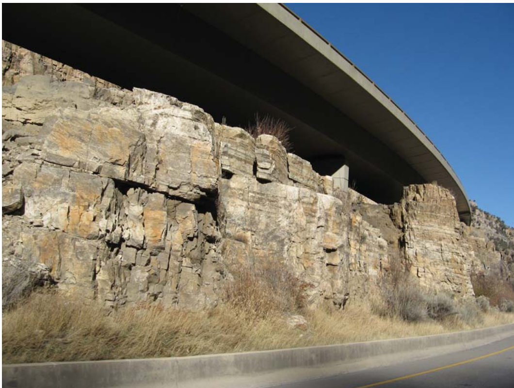
Figure 37. Photo. Staining on the completed cut slope used to create a natural-looking rock face. Glenwood Canyon, Colorado.
