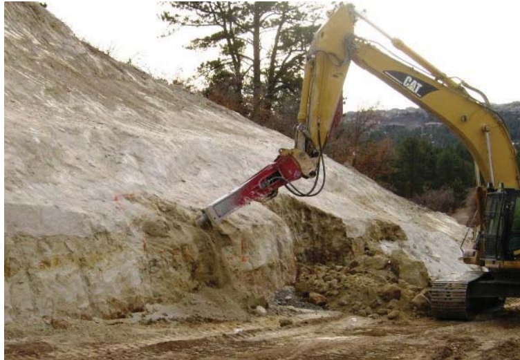
Figure 25. Photo. A hydraulic hammer expanding a sculpted area, creating planting areas and more natural-looking slope variation.
