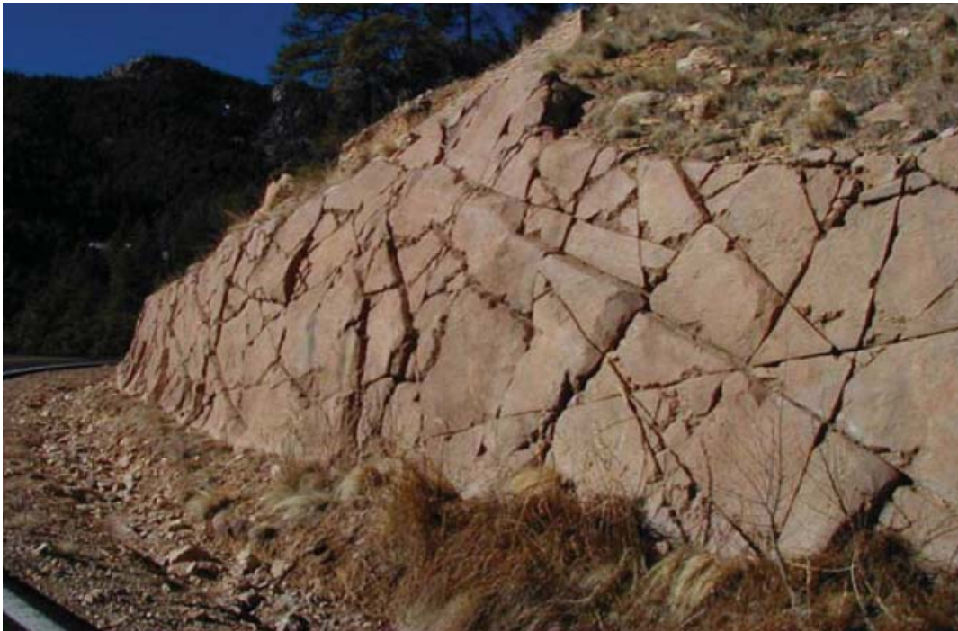
Figure 51. Photo. Shotcrete can be used to protect a slope from erosion—and sculpted to mimic the natural rock face (Ada County Highway District 2003).
