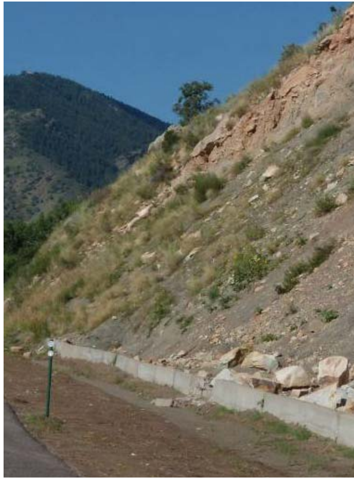
Figure 67. Photo. Concrete barriers used as a rockfall protection measure. Notice the damage caused by a large rock impact.
