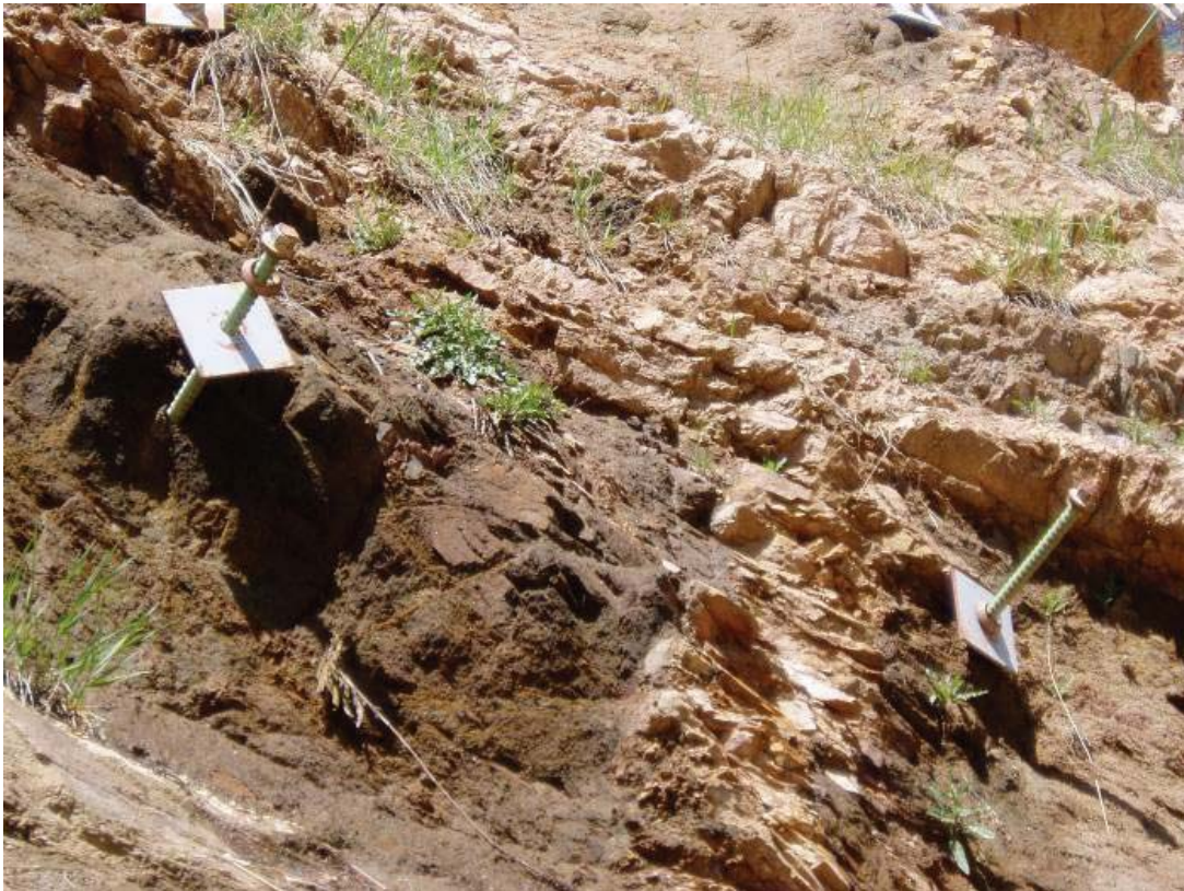
Figure 45. Photo. Rock bolts installed in an area where the surrounding rock has eroded away, reducing the effectiveness of the bolts.
