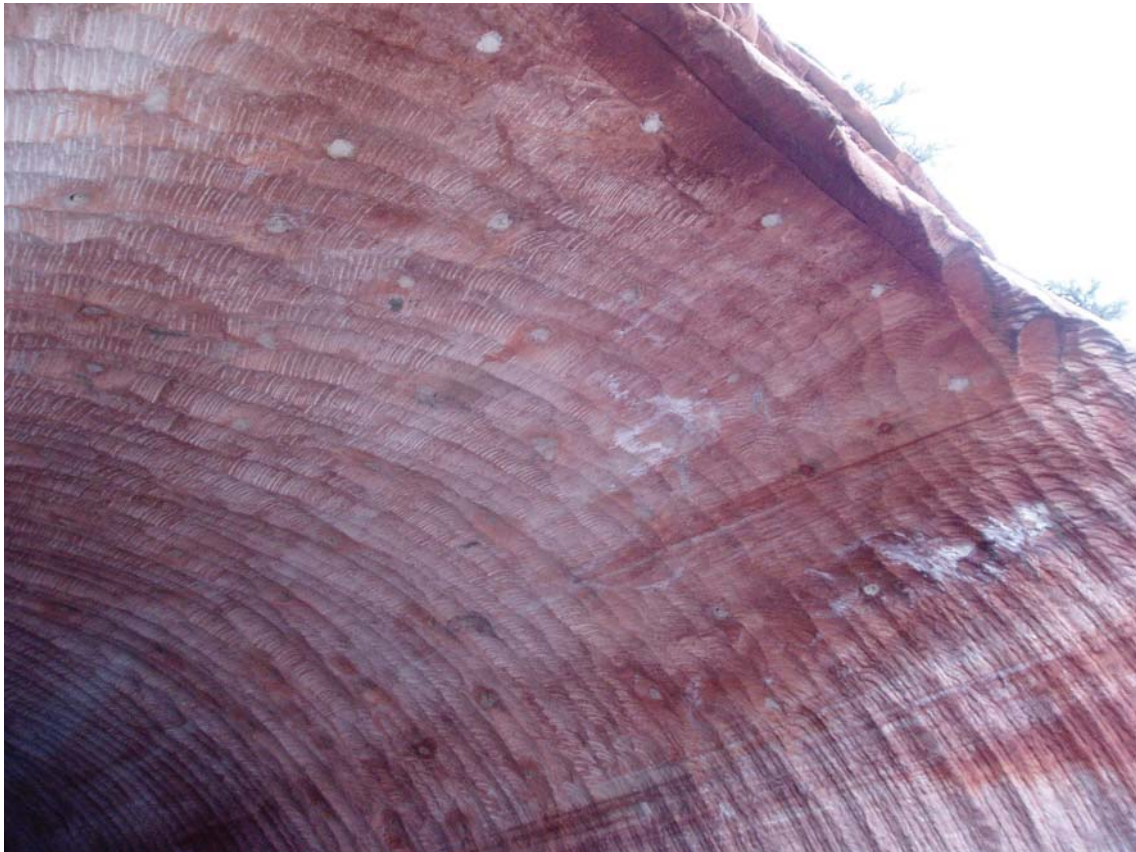
Figure 44. Photo. Tunnel crest supported with dowels that have been covered with colored grout.
