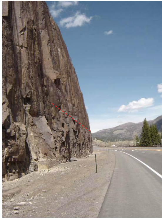
Figure 58. Photo. A rockfall-prone slope draped with unsecured wire mesh. Wolf Creek Pass, Colorado.
