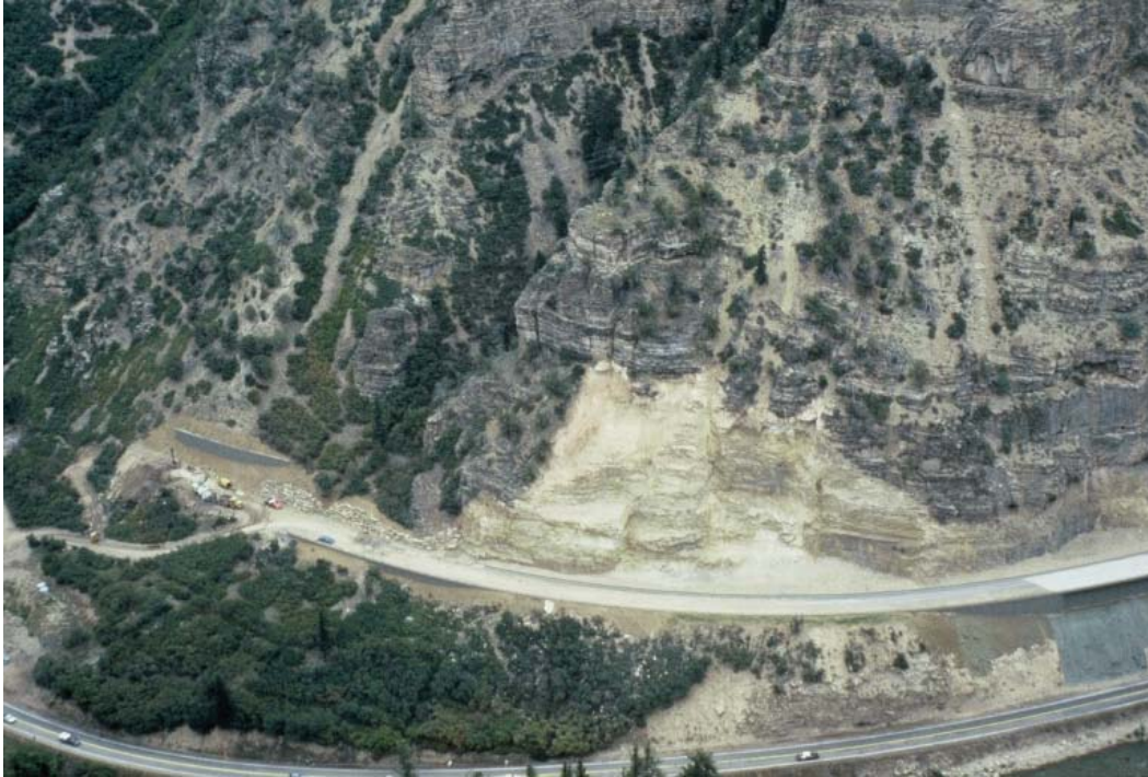
Figure 36. Photo. Rock excavation shortly after construction. Note the stark contrast of the freshly excavated material and the naturally weathered rock surfaces. Glenwood Canyon, Colorado.
