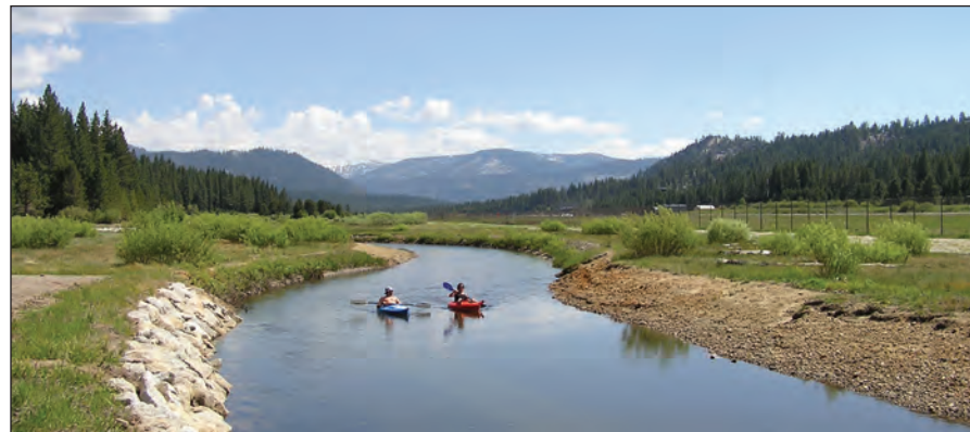
The Upper Truckee River drains a large watershed (map) that starts near Red Lake Peak along Highway 88. Restoration work has included re-meandering the river and stabilizing banks with rock and native plants.
