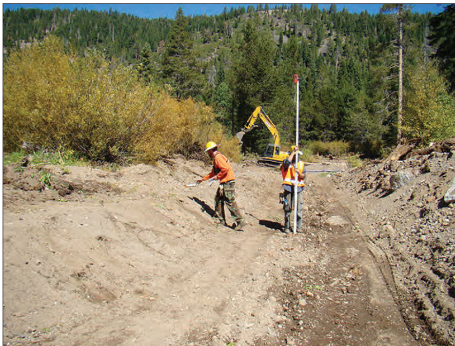
Rebuilding flood-damaged portions of Blackwood Creek involved making careful measurements and using natural materials to deflect stream flows.
