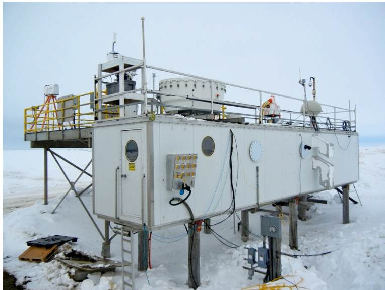
Figure 2. KAZR installation at Barrow.
