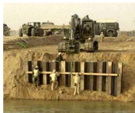
Dr. Rick Olsen and Gerardo Velasquez, GSL, provided guidance on bridge placement and soil stabilization to Navy SEABEES in the weeks leading up to Operation Iraqi Freedom
