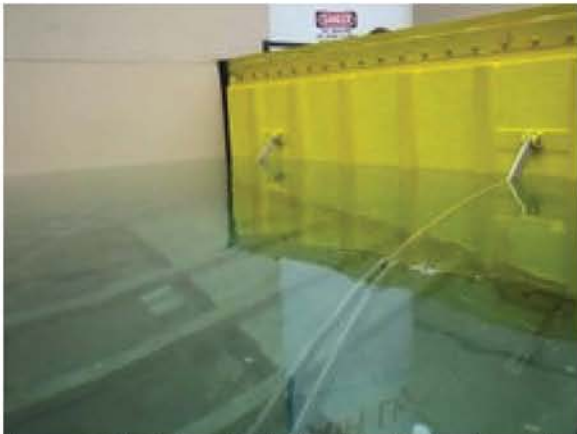
Images of the Automatic flood gate for the Loading dock.
